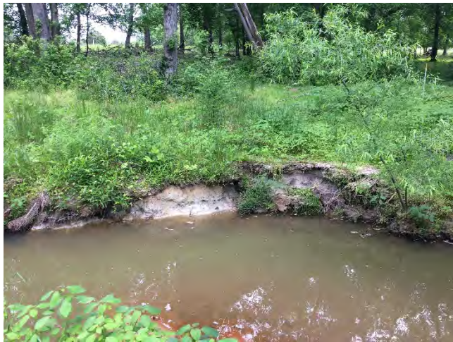
Candy Creek Reach 3 - Bank erosion, RB (Sta. 151+70-152+00) (05/13/2020)
