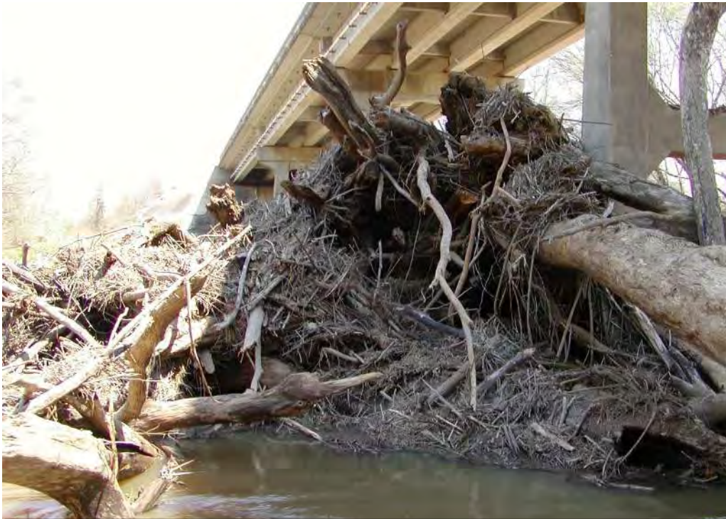
Debris pile accumulated within the Site impoundment that has accumulated against bridge pilings
