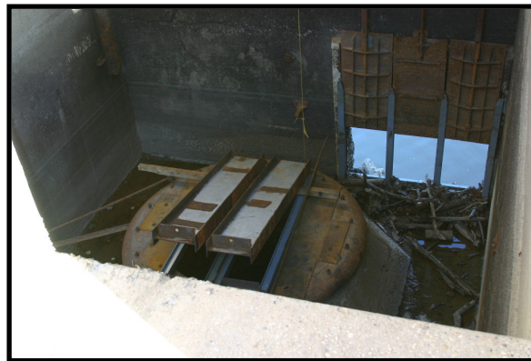
Photo 1: Repaired mud gates and flap covers on draft tube In southern water well Source: Restoration Systems 2005
