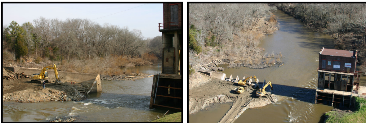
Photos 12 and 13. Two stages of spillway breach to facilitate dewatering Source: Restoration Systems 2006
