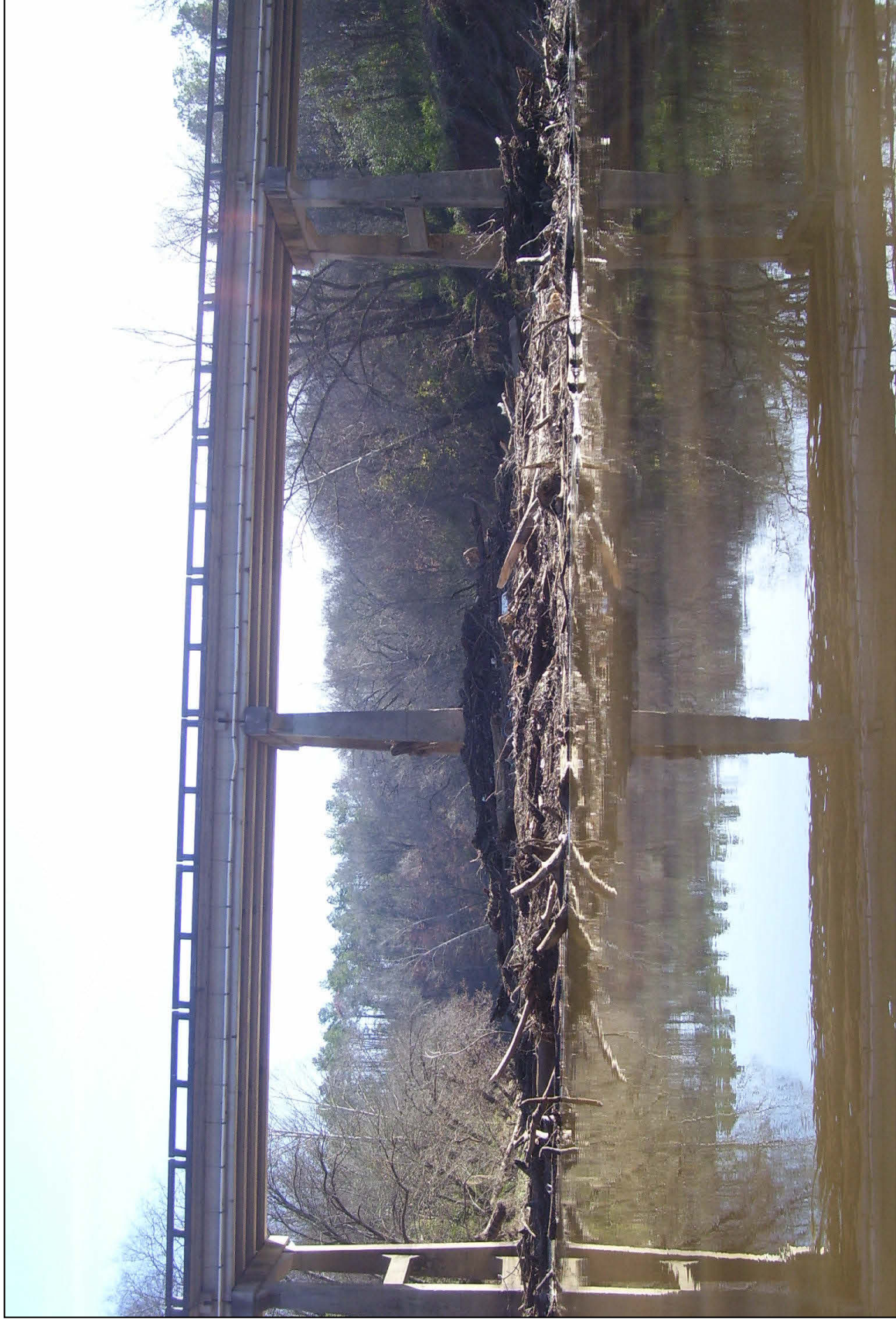
Location: Carleton Road crossing of the Deep River Description: Log jam behind bridge spans
