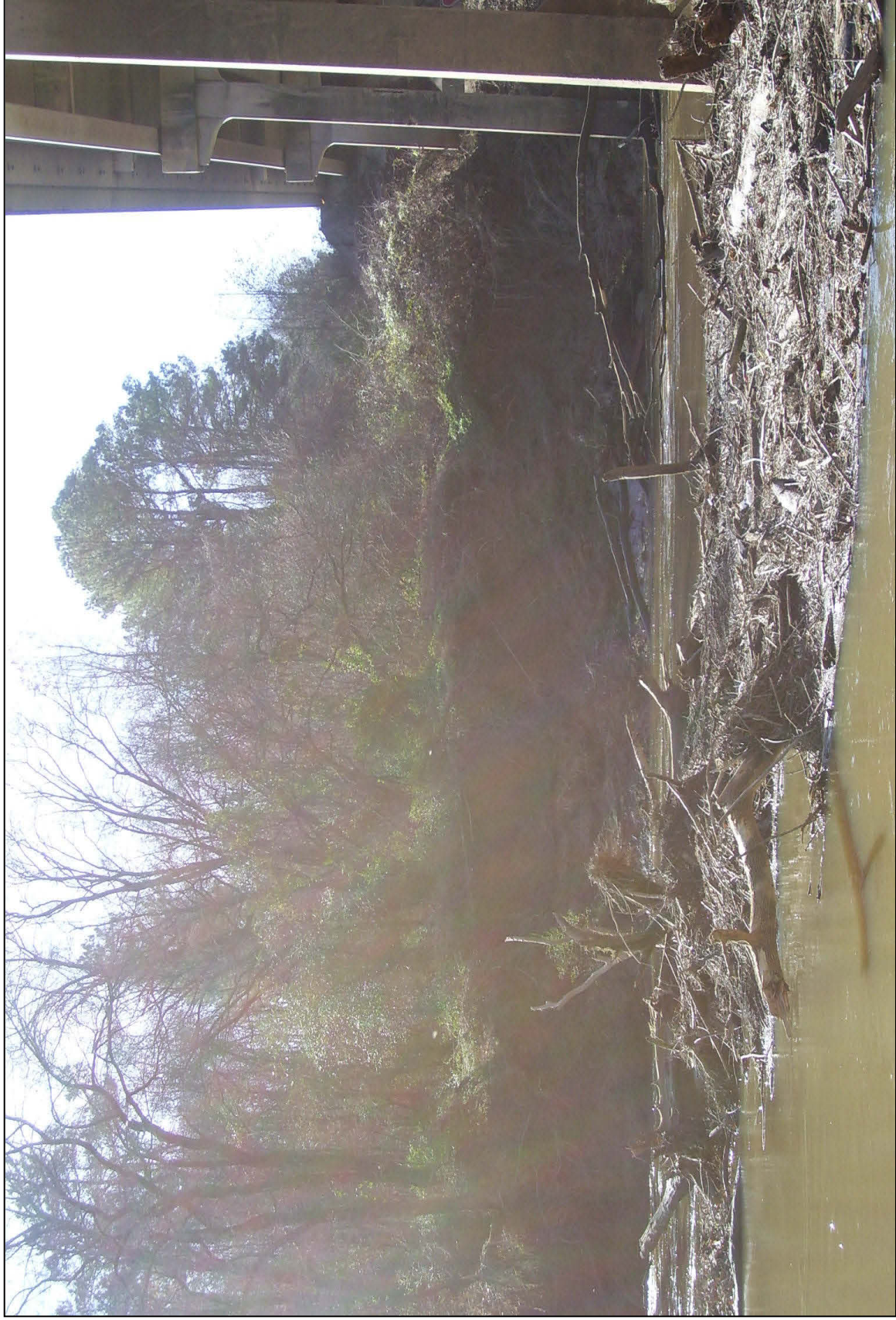
Location: Carabnton Road bridge crossing of the Deep River Description: Sloughing of bank material downstream of the bridge
