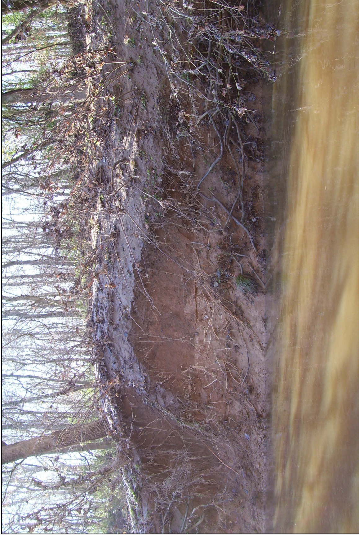
Location: Deep River downstream of the Norfolk-Southern rail bridge Description: Bank failure and continued erosion into the Deep River
