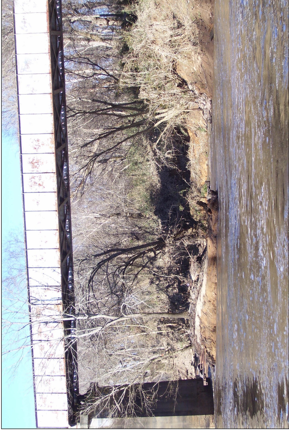
Location: Deep River downstream of the Norfolk-Southern rail bridge Description: Continued bank failure and sloughing into the Deep River
