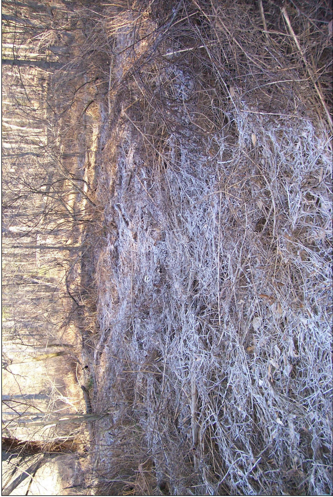
Location: Line Creek upstream of the bridge crossing of Caribton Road Description: Sediment deposition as evidence of overbanking
