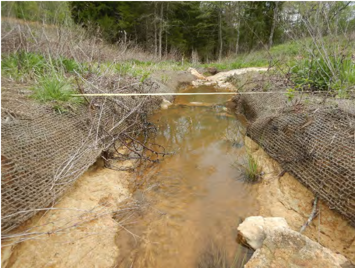
UT1 R3 XS7 downstream – Area of Bedload Movement (Pre-Repair) (04/15/2021)
