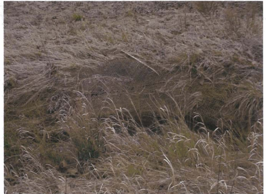
Photo Station 14.A: Looking at erosion hole.
