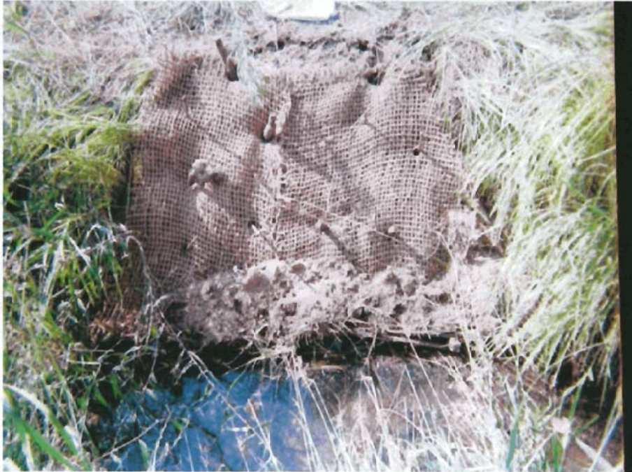
Photo 1: Looking at erosion hole fix upstream of Station 20+00
