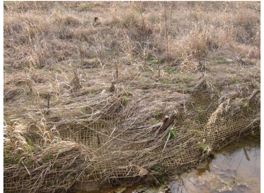
4. Vegetative Cover Poor– 3/30/06
