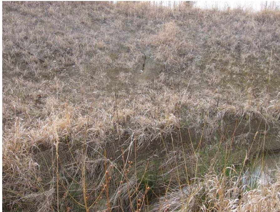
5. Vegetative Cover Poor– 3/30/06
