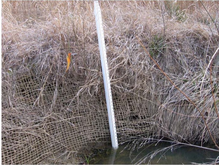
1. Bank Erosion: Moderate– 3/30/06
