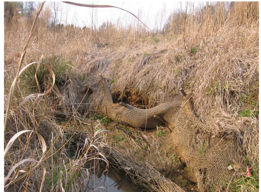
2. Bank Erosion: Severe– 3/30/06
