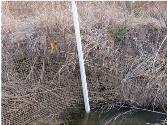
1. Bank Erosion: Moderate – 3/30/06
