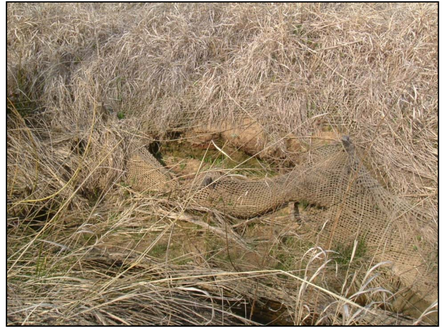
2. Bank Erosion: Severe 3/21/2007
