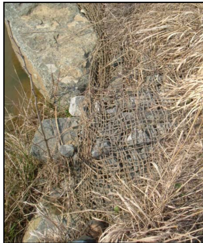
3. Streambank Cover Poor 3/22/2007
