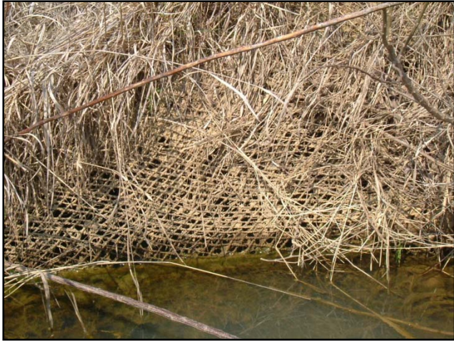
1. Bank Erosion: Moderate 3/22/2007
