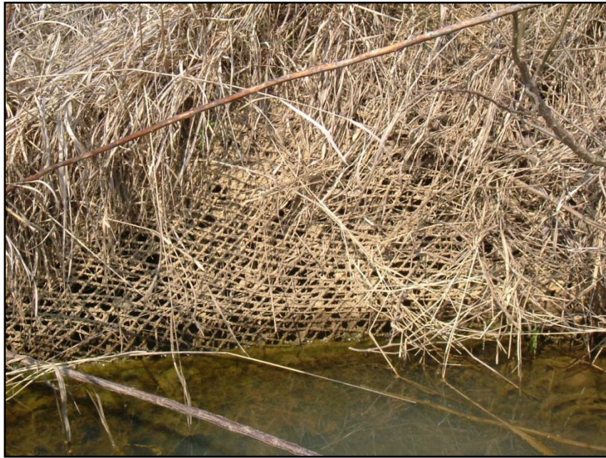
1. Bank Erosion: Moderate 3/21/2007
