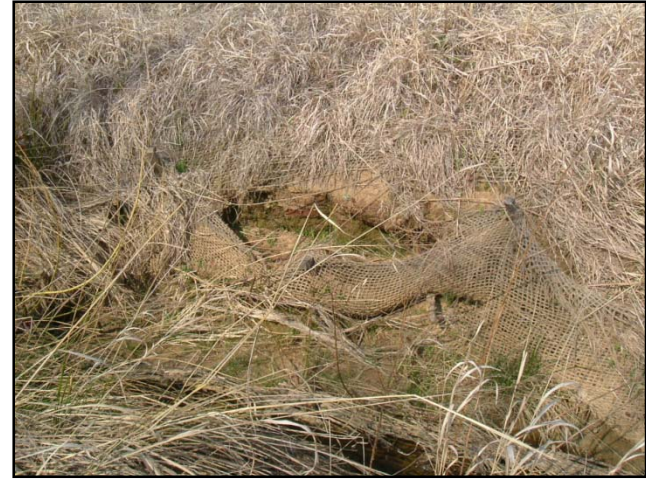
2. Bank Erosion: Severe 3/22/2007
