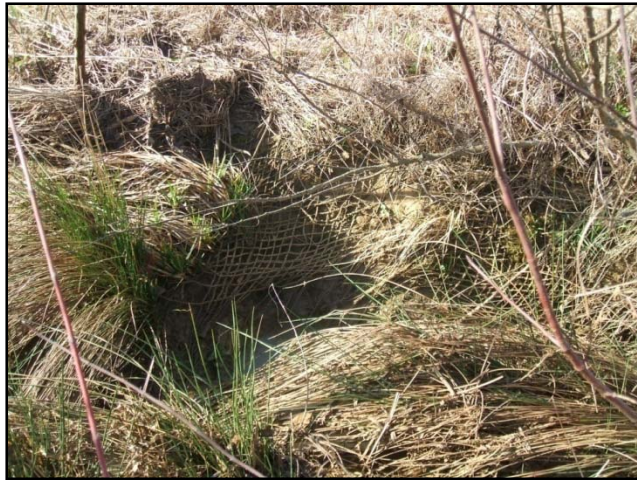
1. Bank Erosion: Moderate (3/2008)
