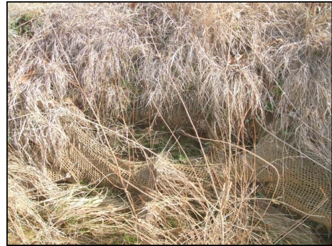
2. Bank Erosion: Severe (3/2008)
