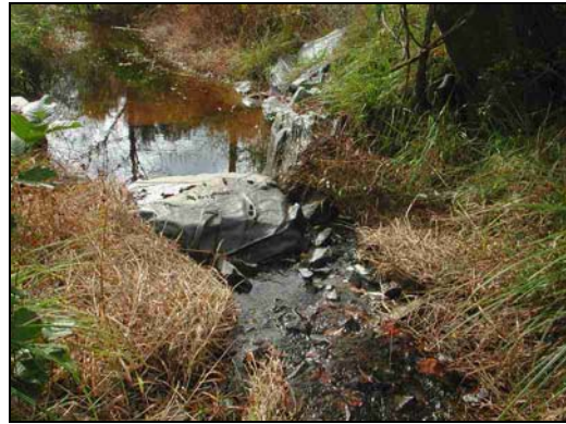
SPA2. Station 10+85: Minor erosion below arm.
