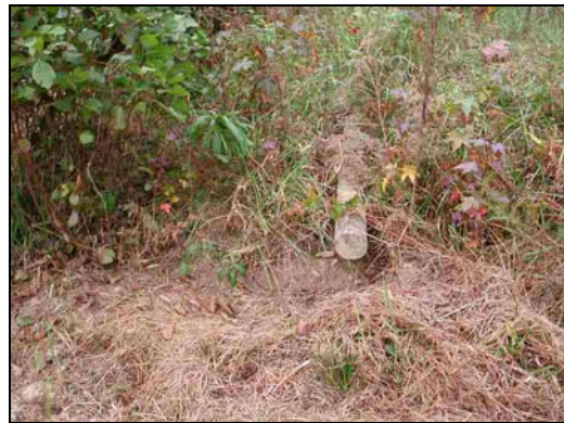
SPA4. Station 18+60. Fence pulled out by stress from debris jam at high flow.
