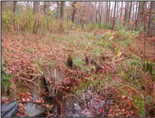
SPA1. Station 27+50 to 27+75: Matting detached DS of cross vane
