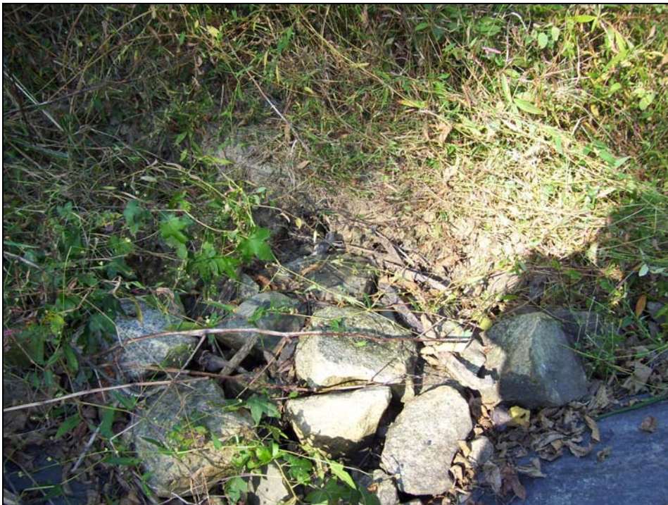
SPA 13. Cross vane failure.
