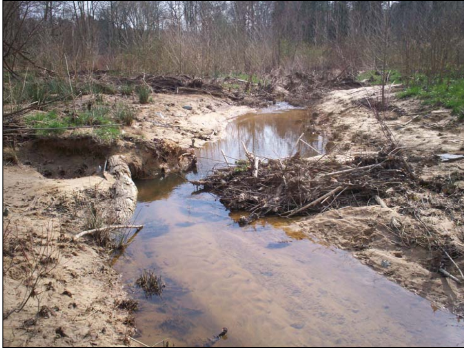
SPA 6. Bank failure behind rock vane.
