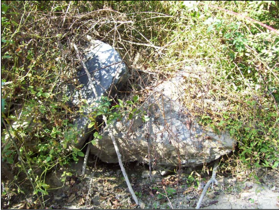
SPA 4. Erosion at cross vane.
