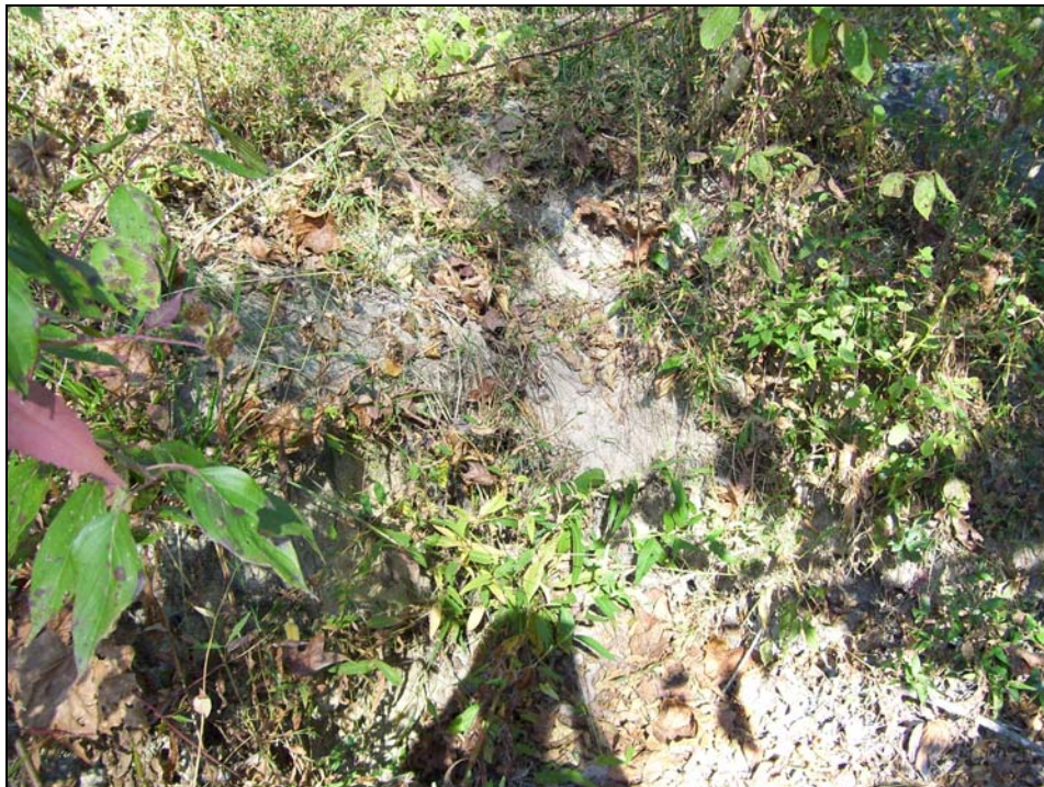
SPA 3. Right bank erosion.
