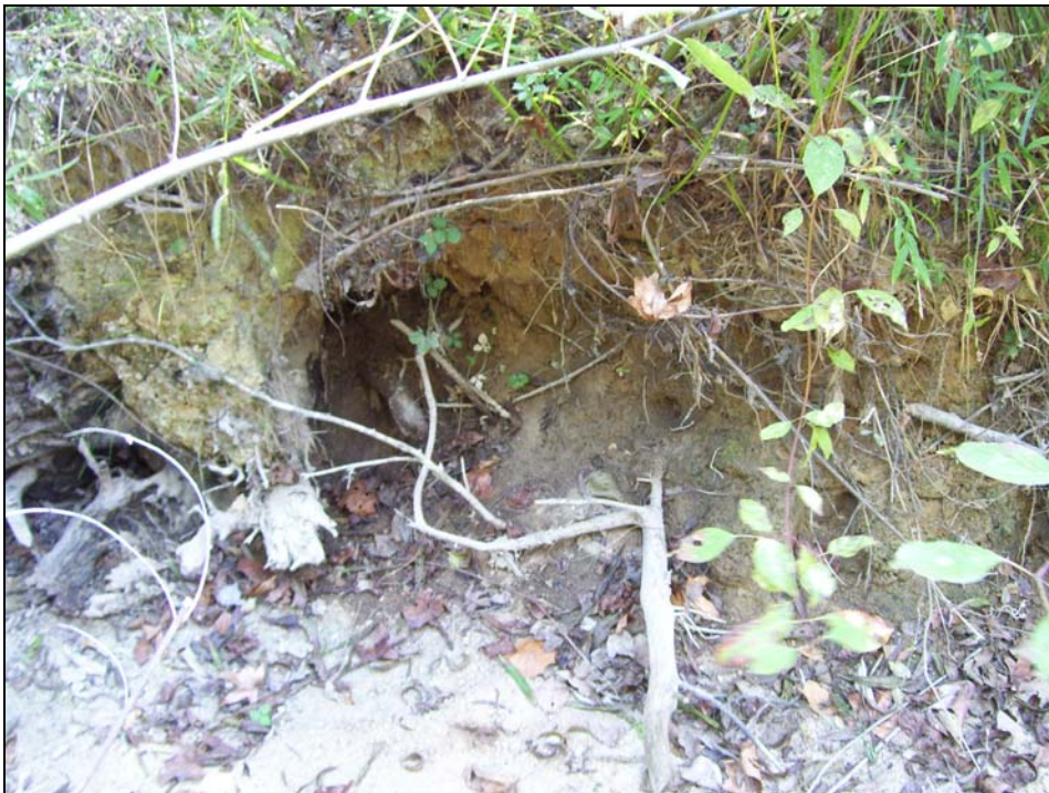
SPA 5. Left bank failure behind rock vane.
