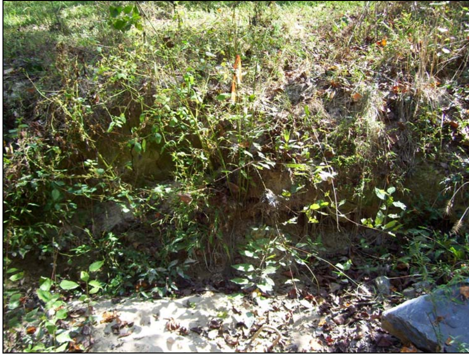
SPA 10. Left bank erosion at cross vane.
