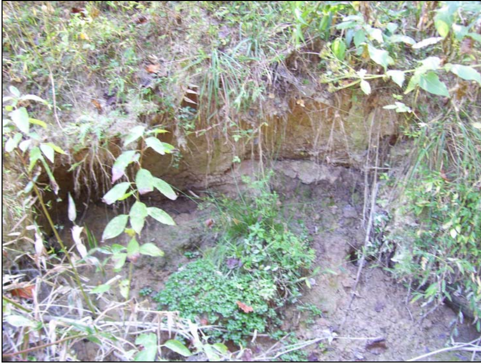
SPA 12. Bank failure at cross vane.
