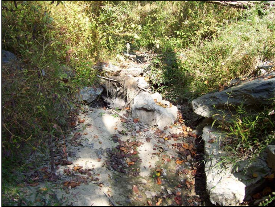
SPA 8. Left bank erosion at cross vane.
