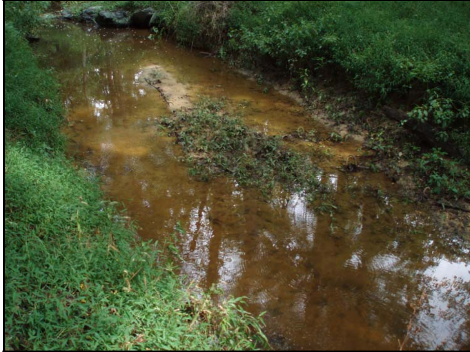
PA #13 – Mid-Channel bar forming. Sta. 27+60
