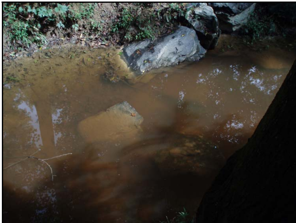
PA #12 – Erosion at J-hook; header rock displaced. Sta. 27+00
