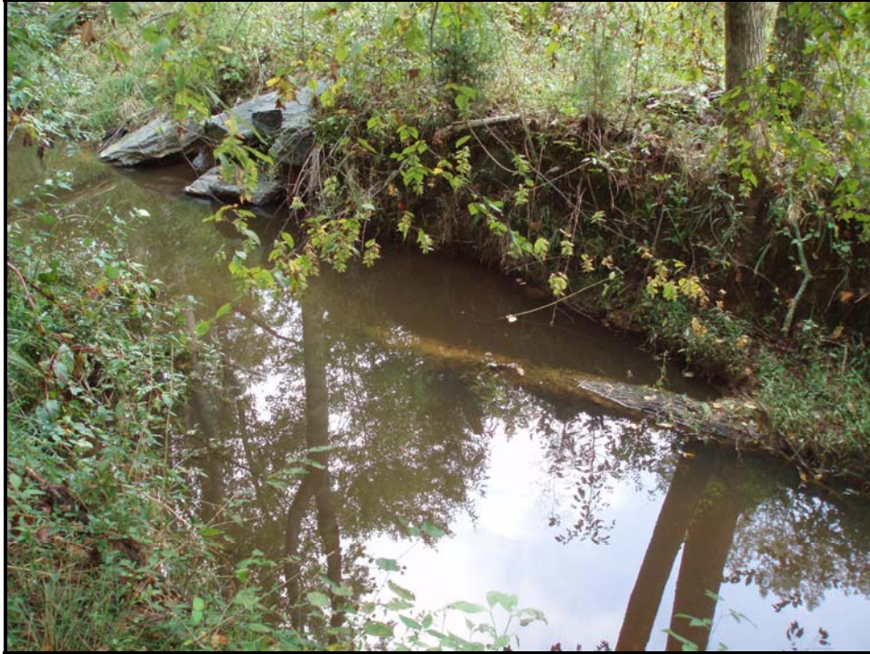
PA #9 – Left bank erosion behind log vane. Sta. 25+00
