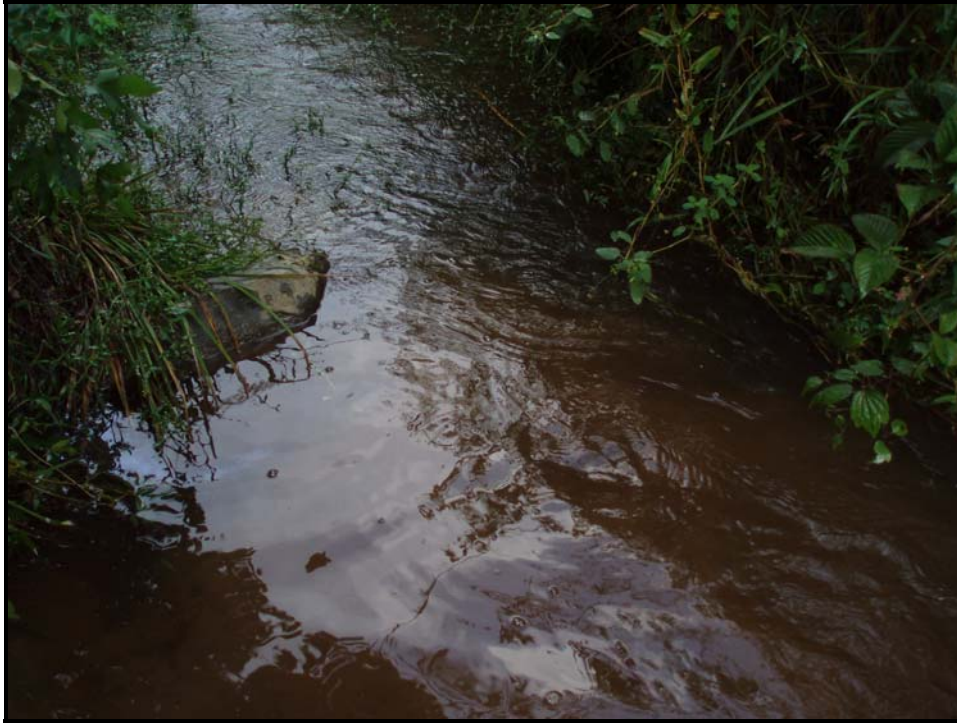
PA #1 – Erosion at cross vane; header rock displaced. Sta. 10+75
