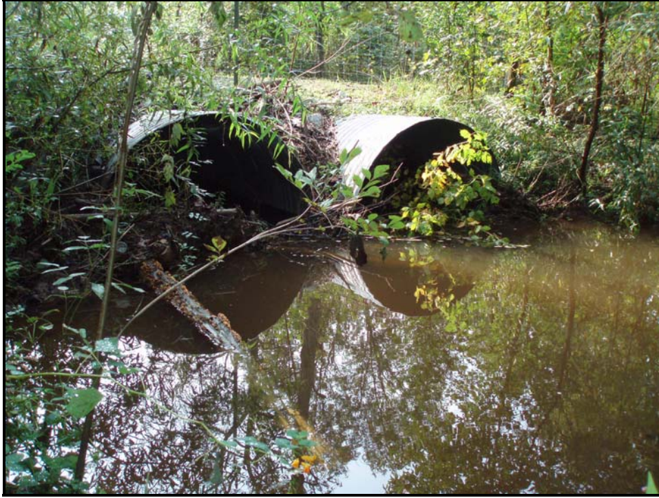
PA #3 – Beaver dam at culvert. Sta. 13+50
