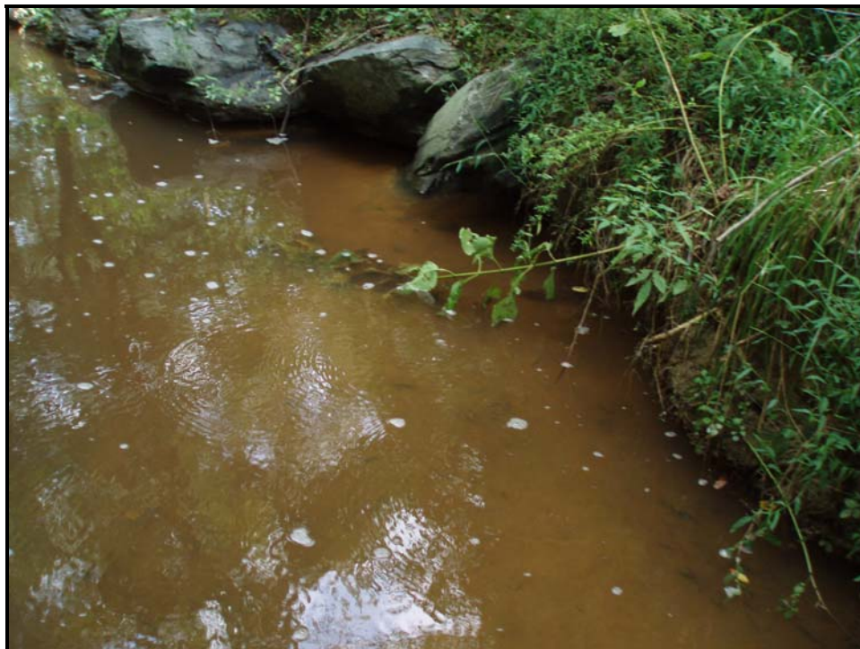
PA #14 – Left bank erosion/undercutting at cross vane. Sta. 27+80
