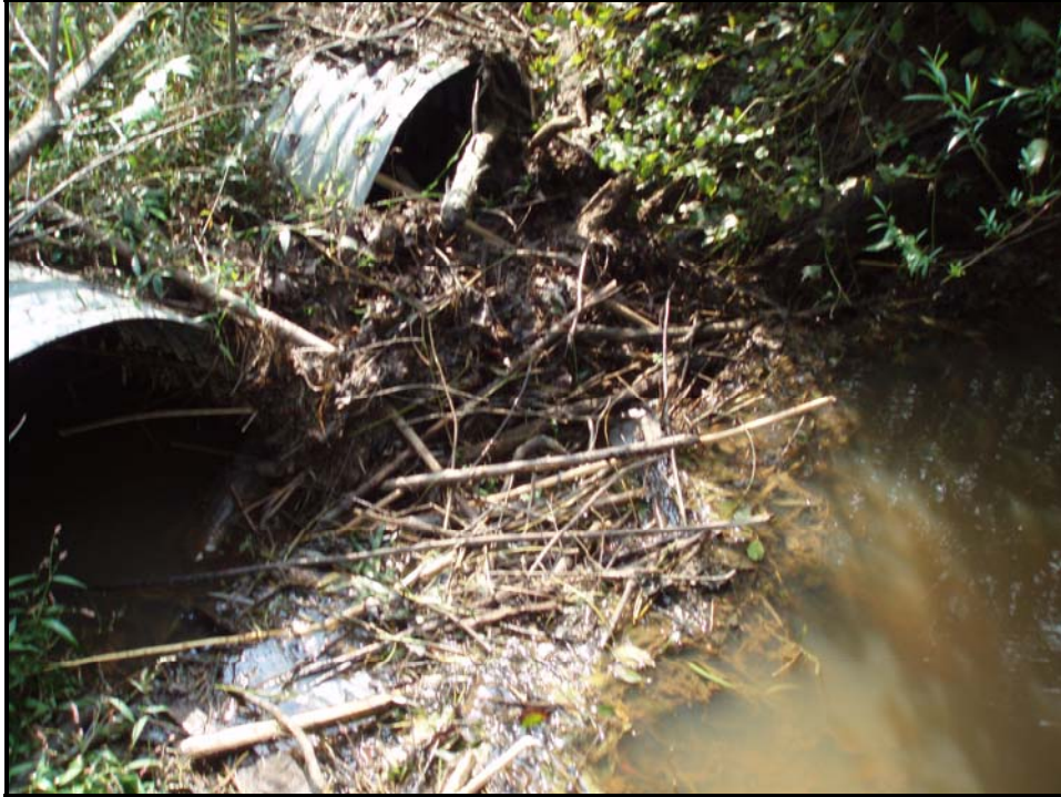
PA #19 – Beaver dam at culvert. Sta. 53+25
