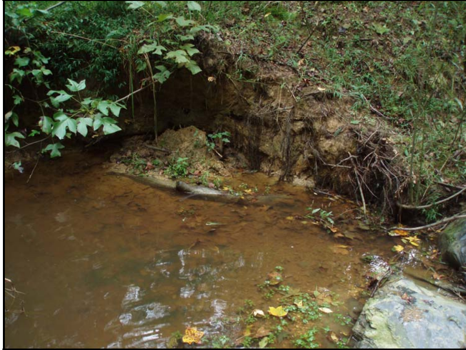
PA #15 – Left bank erosion upstream of cross vane. Sta. 29+40
