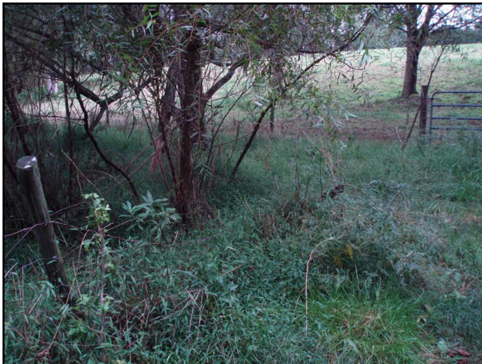
PA#6 – Damaged fence. Sta. 18+50
