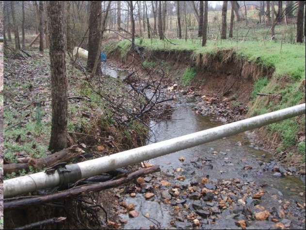
View looking south and downstream at T1. Elevating the channel will increase floodplain connection and hydrology. 3/19/15
