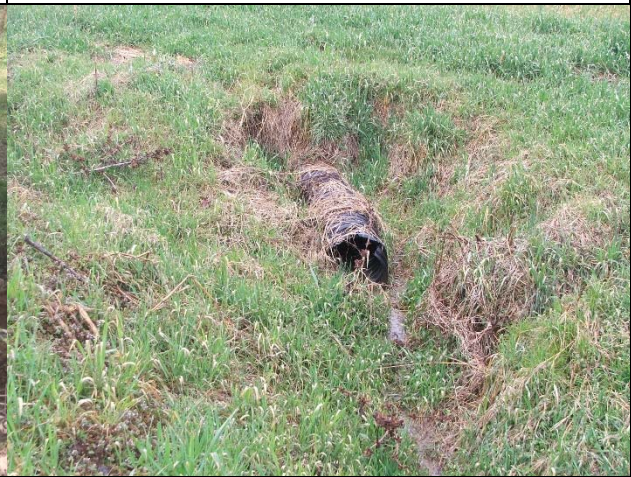
Drain emptying into the top of T3. On-site drainage will be directed into BMP's to mitigate nutrient and soil loading. 3/19/15
