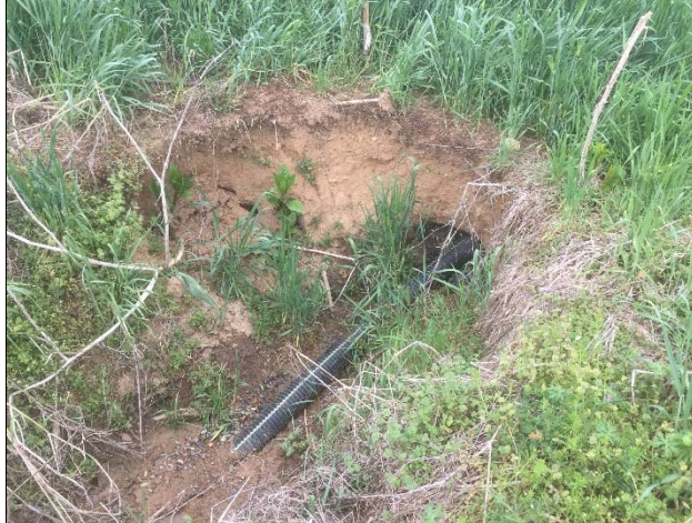
Tile drain emptying into T4. On-site drainage will be directed into BMP's to mitigate nutrient and soil loading. 4/13/15
