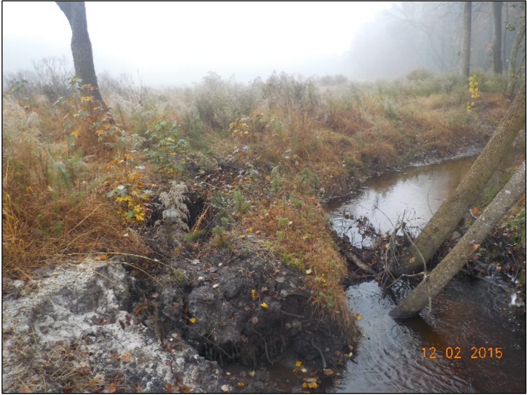
SPA1- Bank Failure @ Sta 25+00 to 25+50
