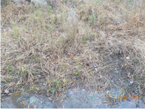
Bank Pin Array at Cross Section 24 (12/02/2015)
