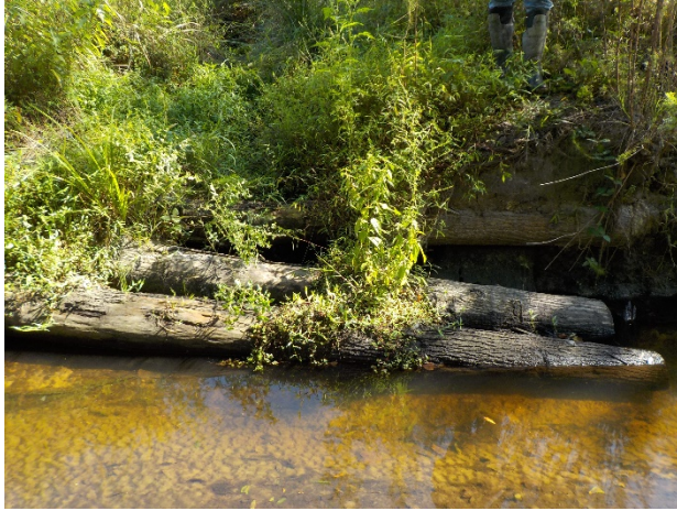
SPA1-Non-functioning Log Outlet Structure – Confluence of UT1 and UT2
