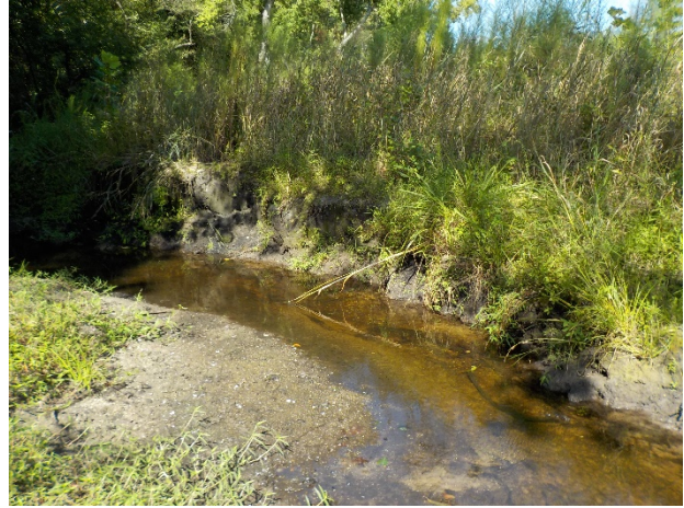
SPA2- Bank Erosion on right bank - UT1 @ Sta. 25+75
