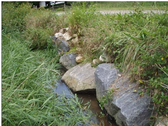
Problem area 1, sta. 1+50, upstream to downstream, 2007.
