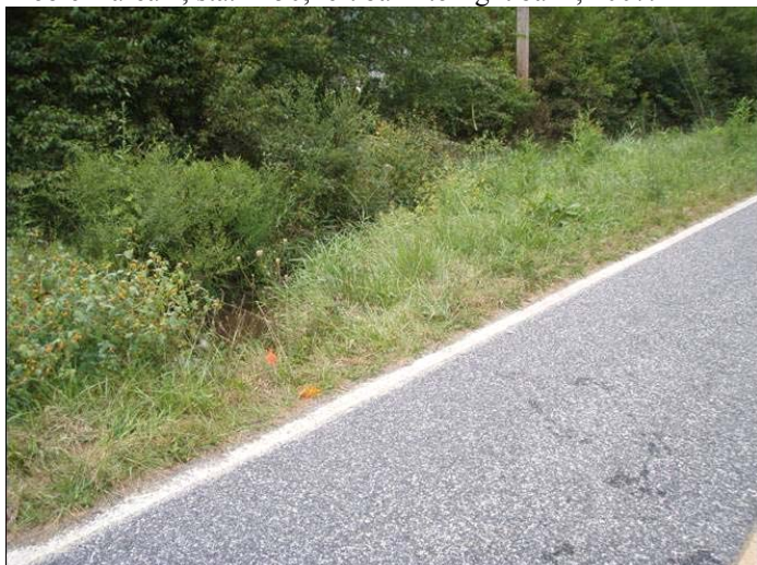
Problem area 1, sta. 1+50, right bank to left bank, 2007.
