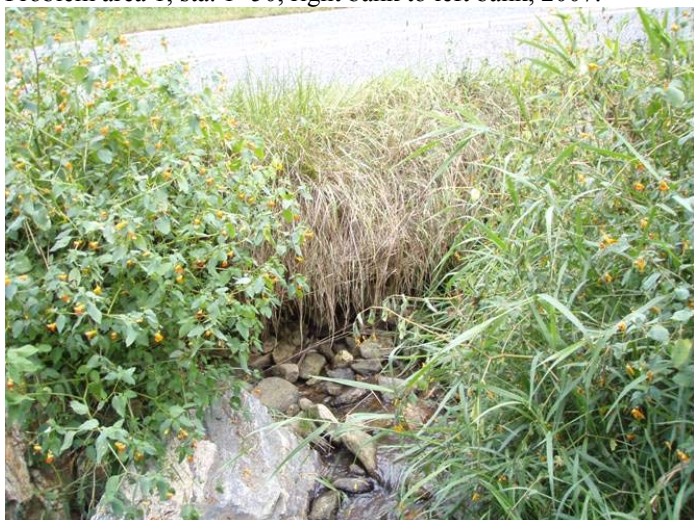
Problem area 1, sta. 1+50, left to right bank, 2007.
