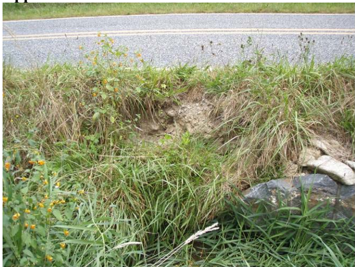
Problem area 1, sta. 1+50, left bank to right bank, 2007.
