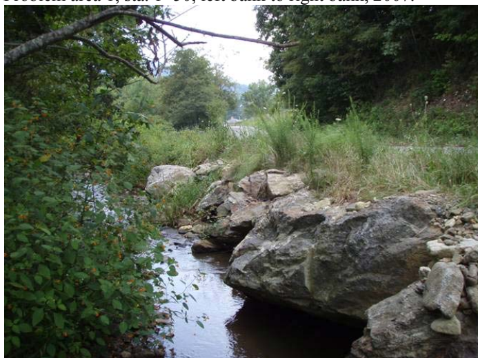
Problem area 2, sta. 5+99, upstream to downstream, 2007.
