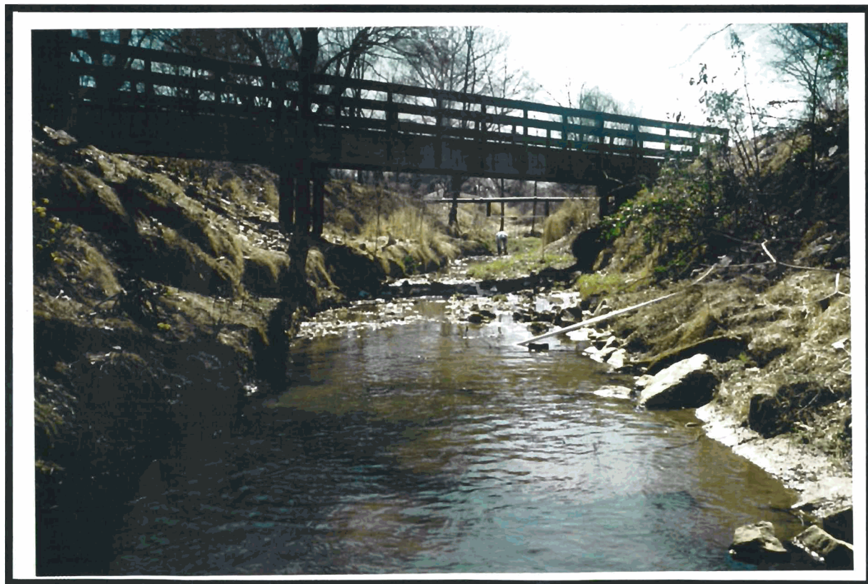
Over Widened Stream Segment Just Downstream of the Culvert
