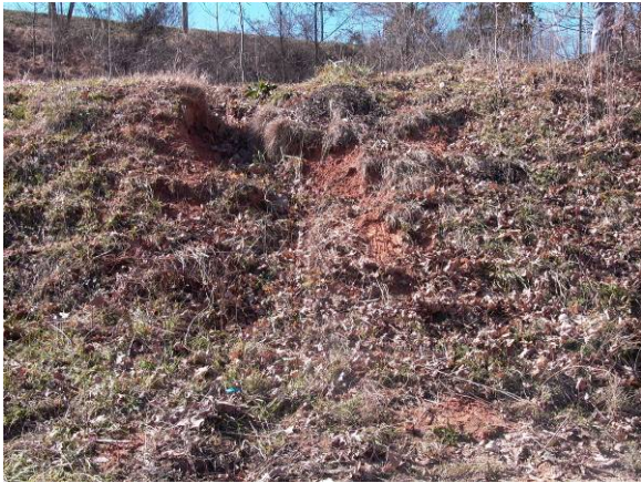
Issue Photo 5 Hillslope Gully erosion At STA: 17+00
