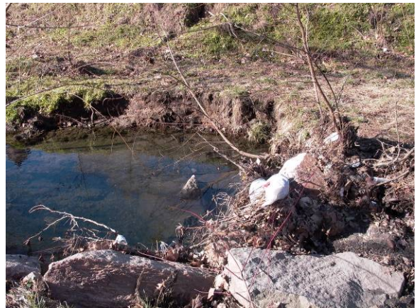
Issue Photo 2. Bank Erosion Due to Urban Debris Blockage
