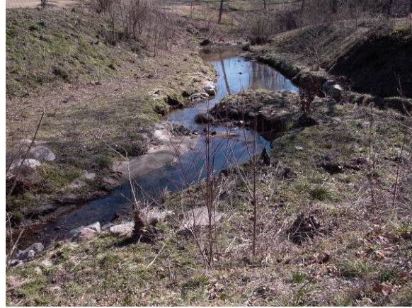
Issue Photo 4 Bank Erosion at STA: 14+75
