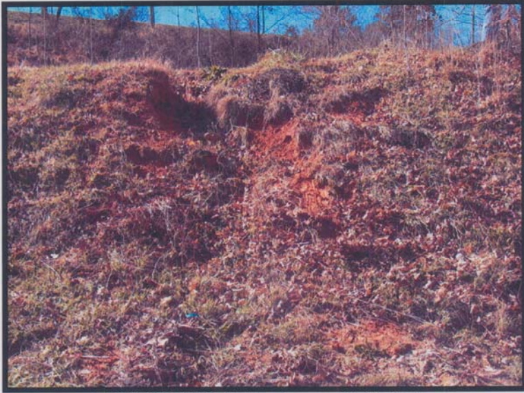
STA 17+00 Gully Erosion on Right Bank
