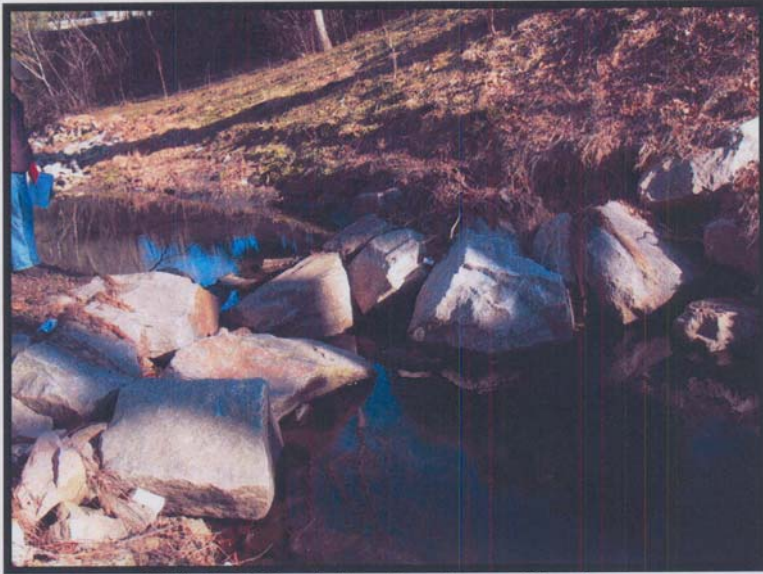
STA 0+95 Bank Arm Erosion on Structure
