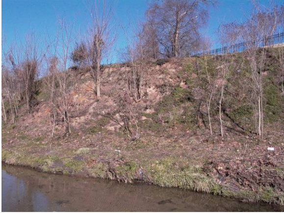
Issue Photo 3 Hillslope Sheet/rill erosion At STA: 15+50 & 16+50
