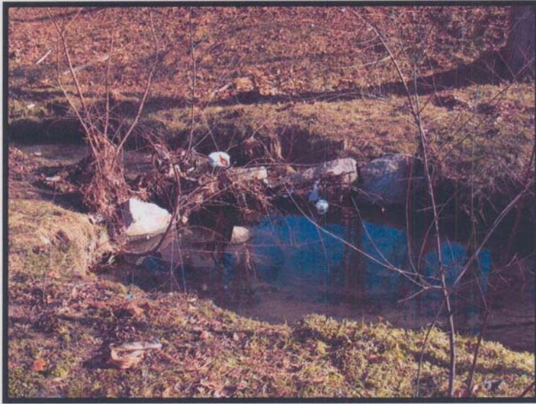
STA 4+75 Blow Out and Bank Erosion
