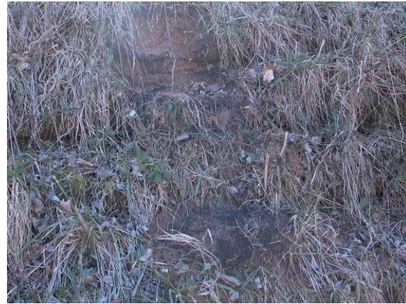
Issue Photo 6 Geo-Grid brake-down at STA: 15+00 on right bank of UT
