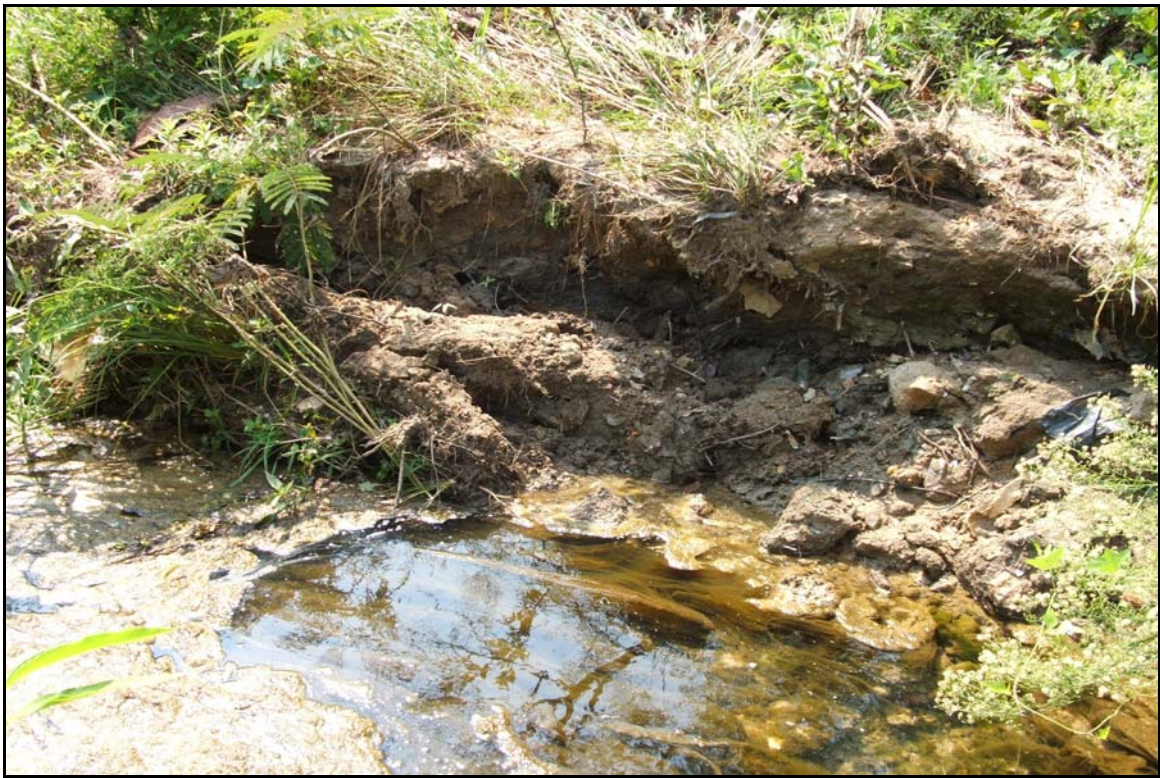
SP2 – Bank erosion/slumping. Photo taken near station 24+50. 8/16/05 - MY 02
