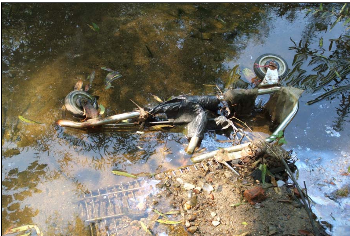
SP4 – Excessive trash, shopping cart and caught trash and debris filling pool. Photo taken near station 14+40. 8/16/05 - MY 02
