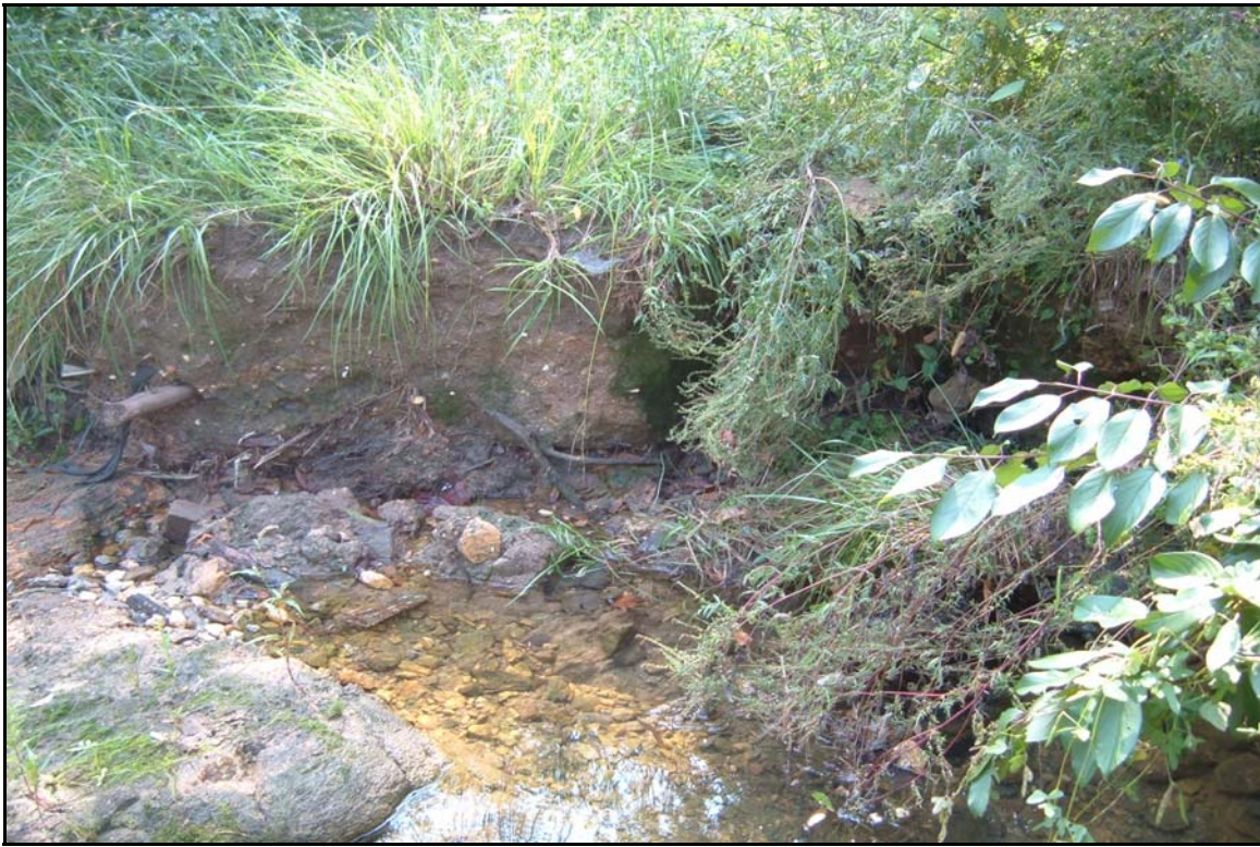
SP2 – Bank erosion/slumping. Photo taken near station 24+50. 10/3/06 - MY 03
