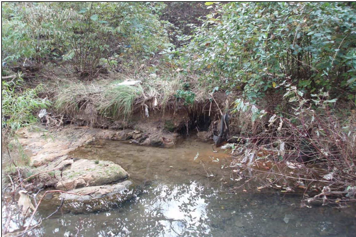
SP6 – Bank erosion/slumping. Photo taken near Station 24+60. 11/12/07 - MY 04
