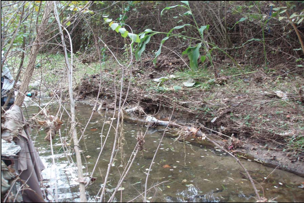
SP5 – Bank erosion/slumping. Photo taken near Station 24+25. 11/12/07 - MY 04
