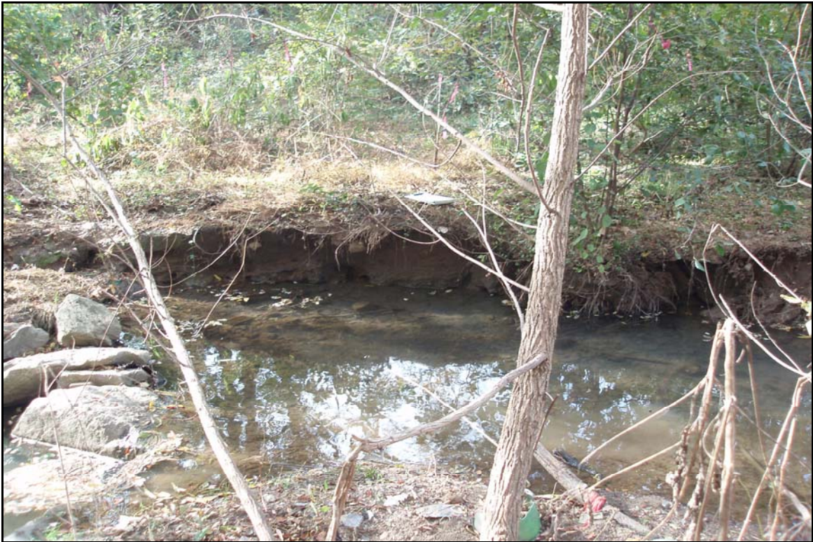
SP4 – Bank erosion/slumping. Photo taken near Station 14+95. 11/12/07 - MY 04
