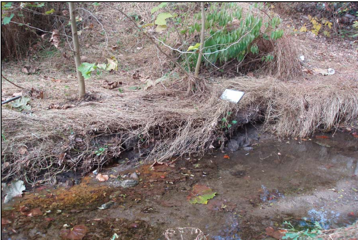
SP2 – Bank erosion/slumping. Photo taken near Station 11+60. 11/12/07 - MY 04
