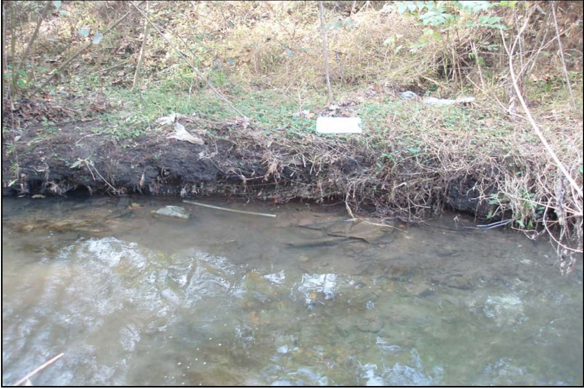
SP3 – Bank erosion/slumping. Photo taken near Station 13+70. 11/12/07 - MY 04
