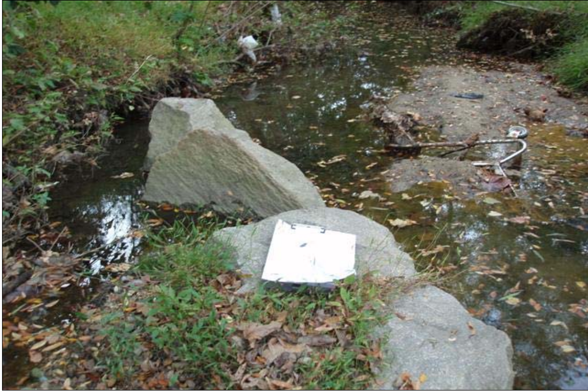
SP3 – Back arm scour, pool aggradation and debris in stream. Photo taken near station 14+75. 10/27/08 - MY 05
