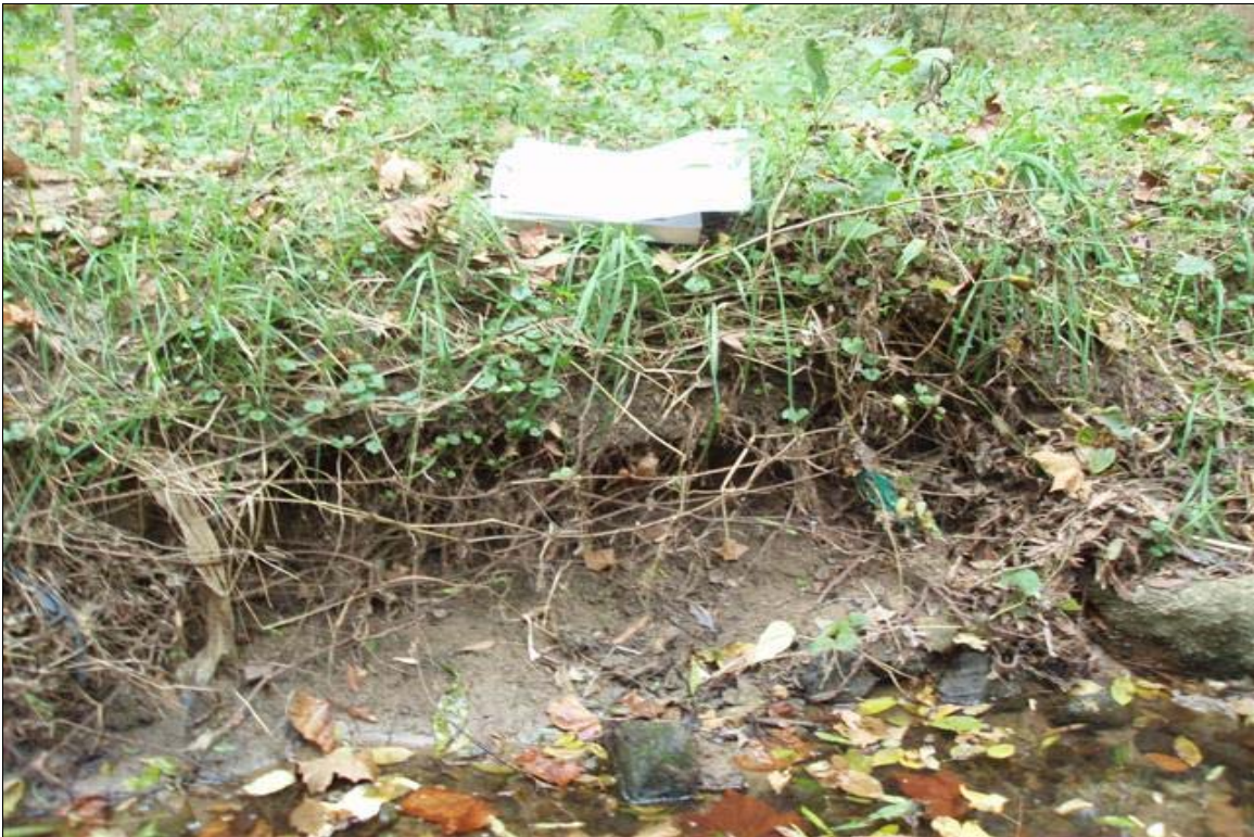
SP2 – Bank erosion/slumping. Photo taken near Station 20+75. 10/27/08 - MY 05
