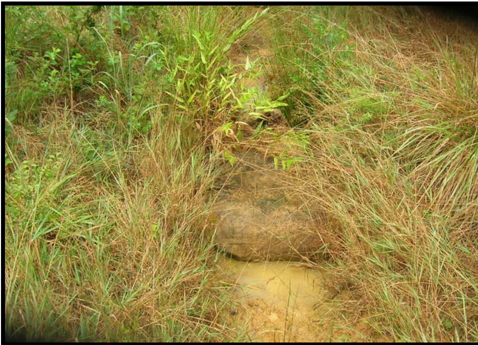
Erosion behind log weir @ station 12+00 (S1)
