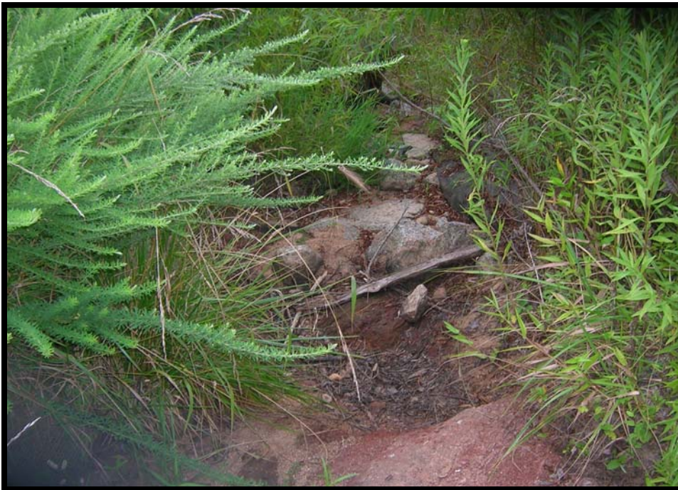
Left bank erosion @ station 10+20 facing downstream (R1)
