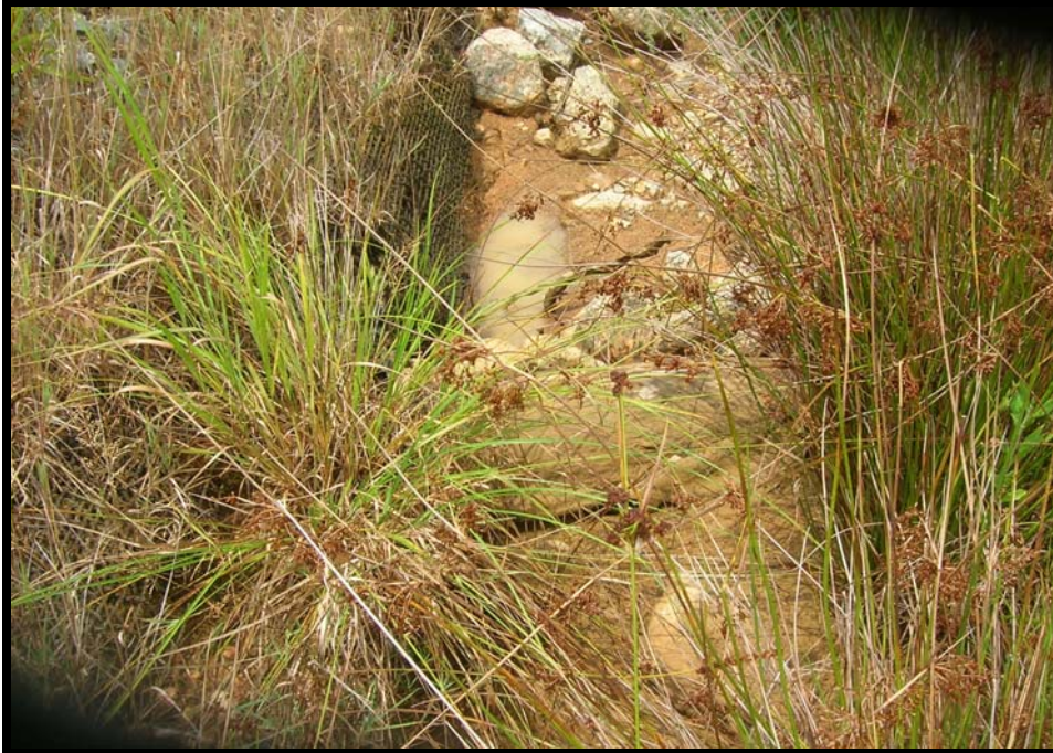
Erosion behind log weir @ station 11+20 (S1)
