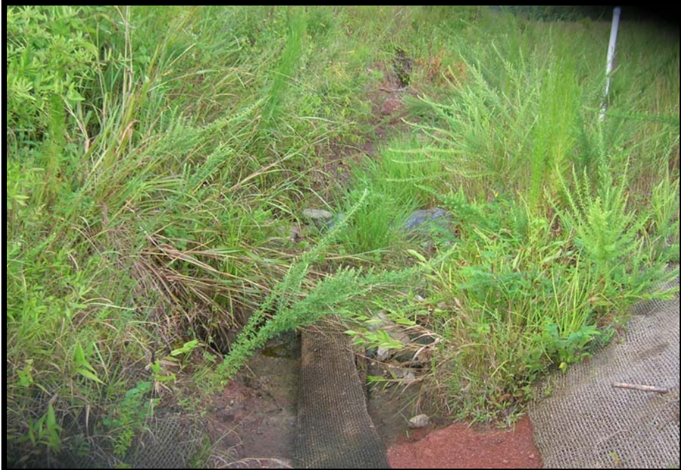
No vegetation along bank @ station 17+00 (R2)
