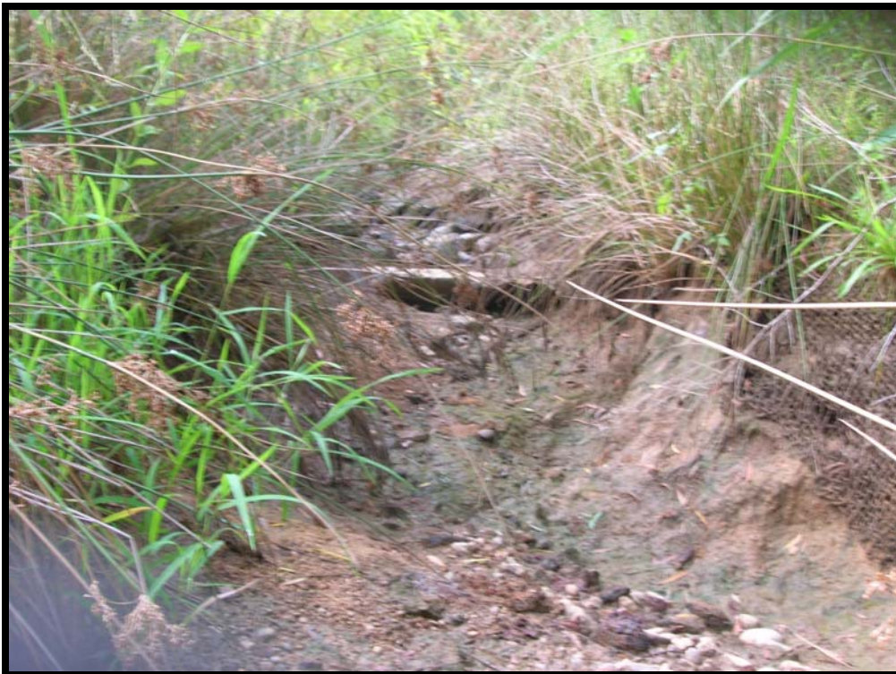
Erosion behind coir matting @ station 36+00 (R2)
