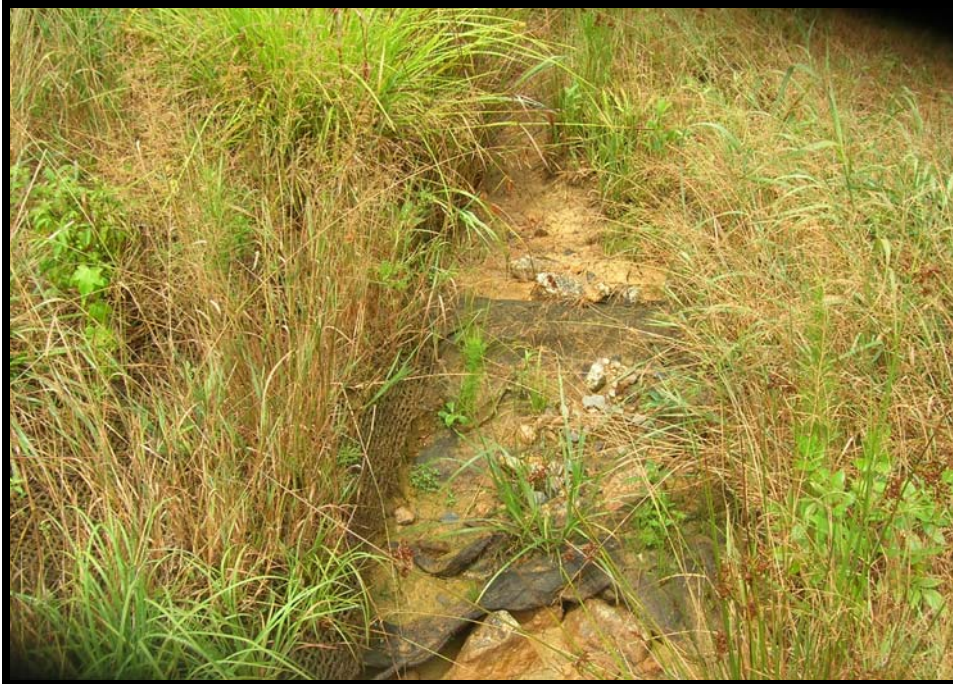
Improper installation of coir matting along Reach R1
