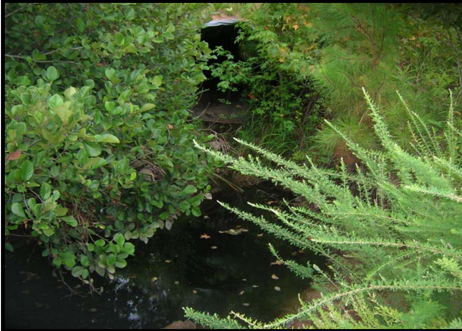
Left bank erosion @ station 10+20 facing upstream (R1)
