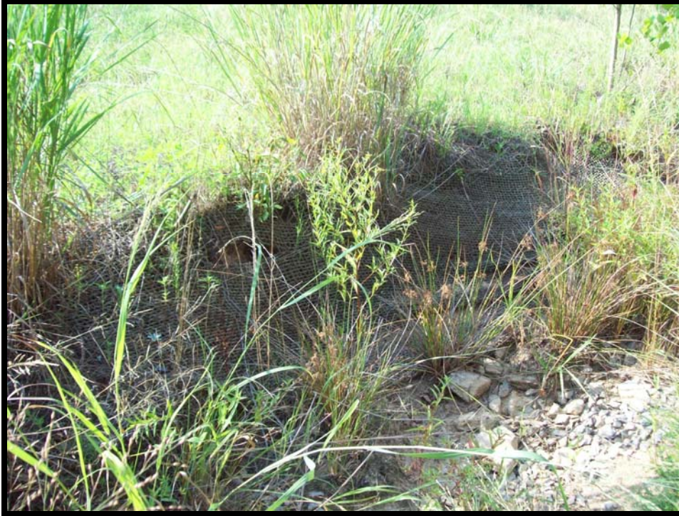
Erosion on left bank @ station 13+20 (S3)
