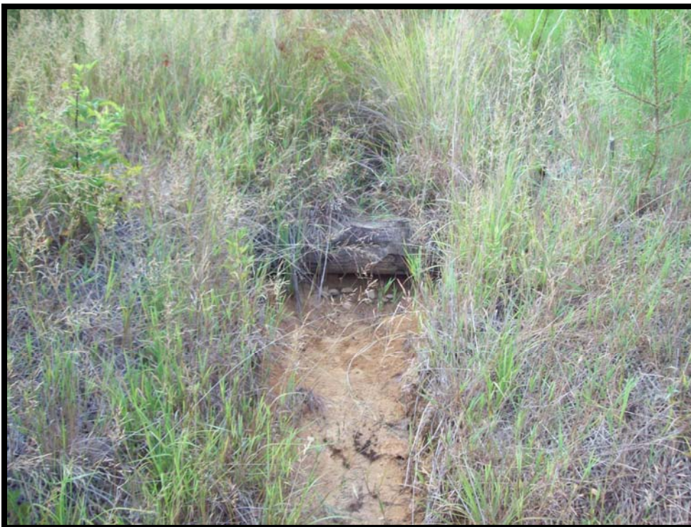
Headcut forming downstream of log weir @ station 15+30 (S1)
