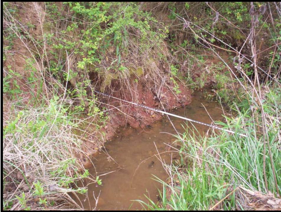
Undercutting along left bank @ station 23+90 (R2)
