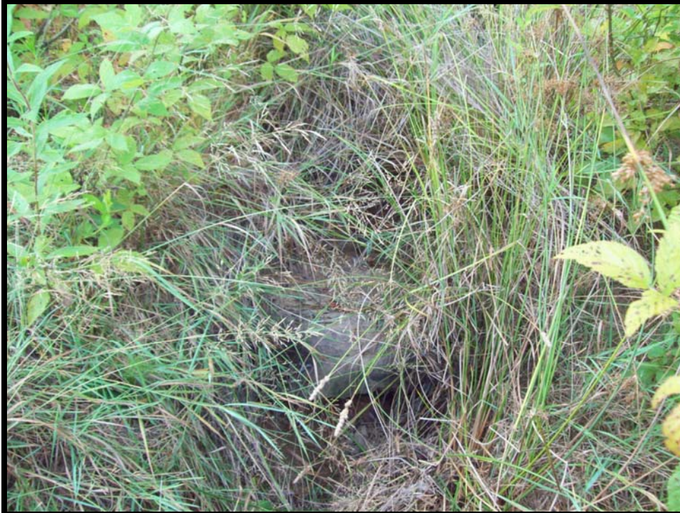
Erosion behind log weir @ station 11+80 facing upstream (S1)
