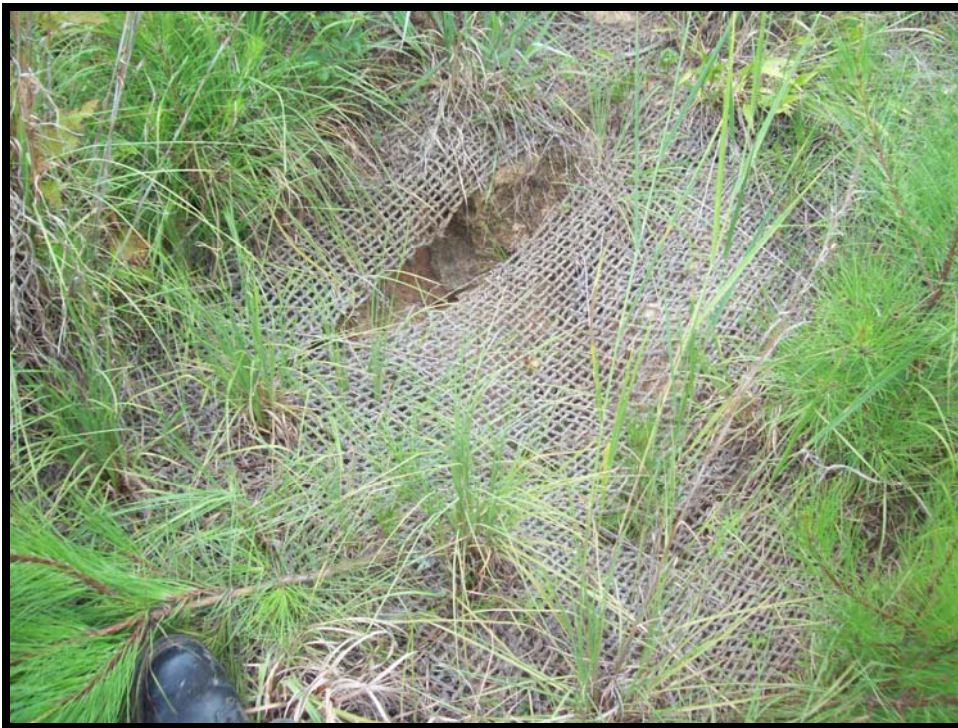
Erosion behind coir matting @ station 18+50 (S5)
