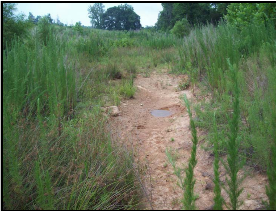
Bare floodplain due to lack of vegetation @ station 48+50 (R3)
