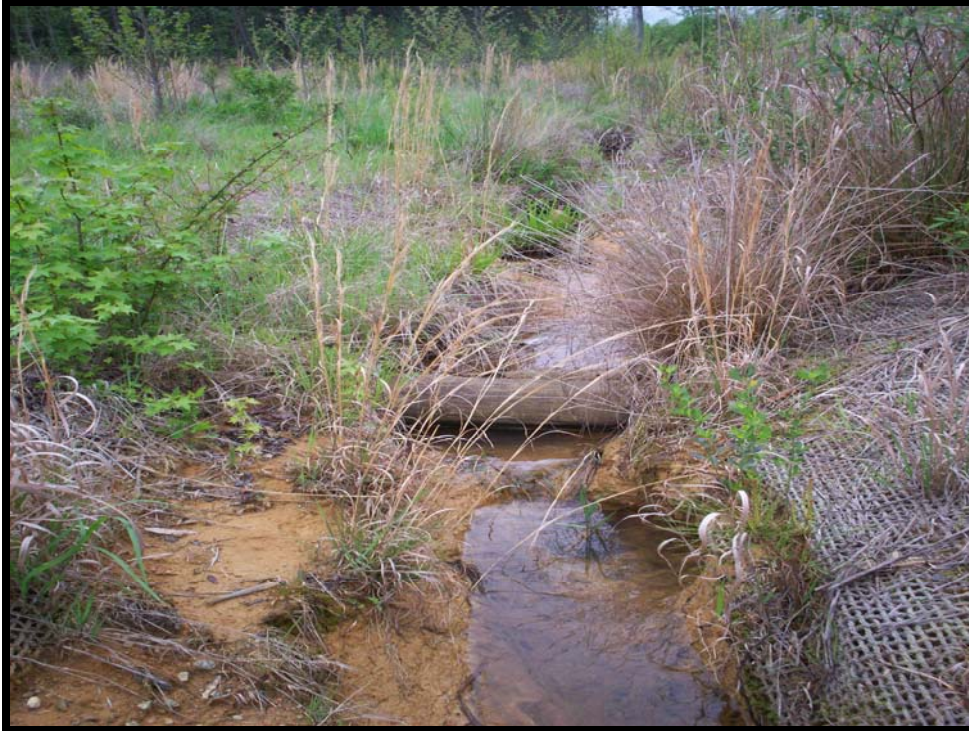
Channel erosion downstream of log weir @ station 15+80 (S1)
