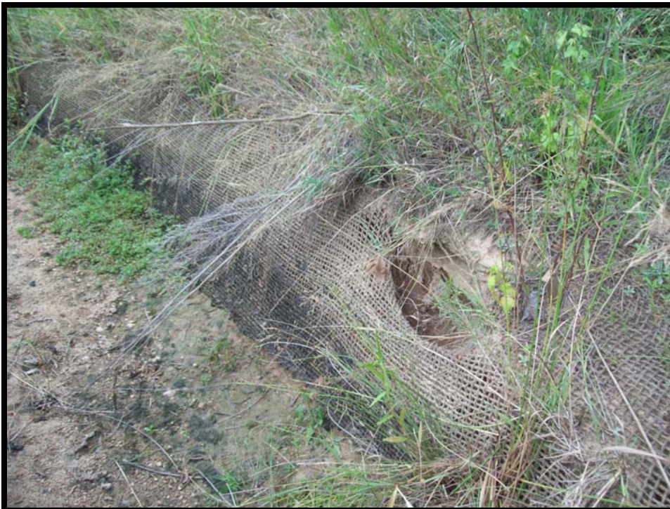
Erosion behind matting along right bank @ station 34+50 (R2)
