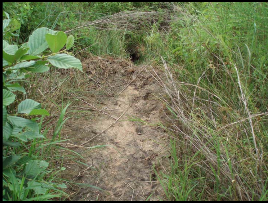
SPA7 - Beaver dam across channel @ station 38+20 (R2)
