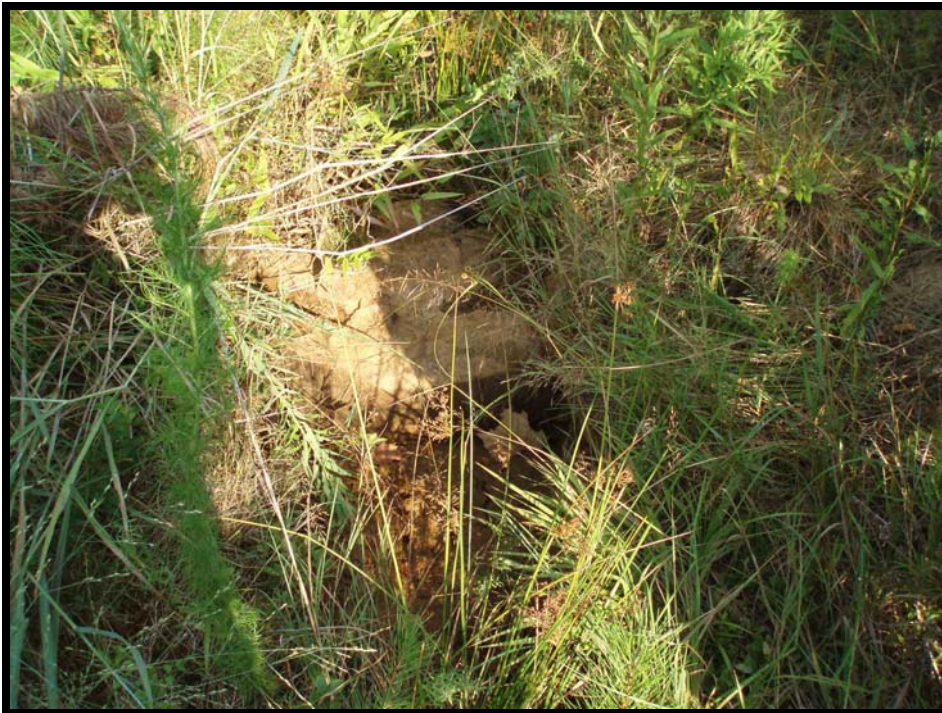
SPA9 - Erosion behind log weir structure @ station 12+00 (S1)
