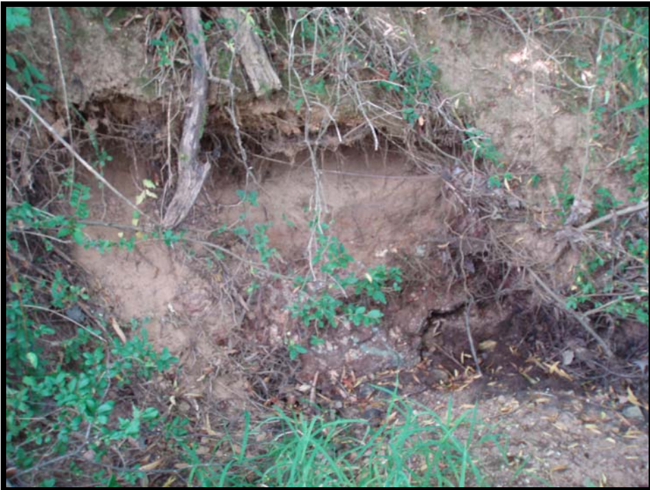
SPA2 - Left bank erosion and lack of vegetation from station 13+80 to 14+10 (R1)
