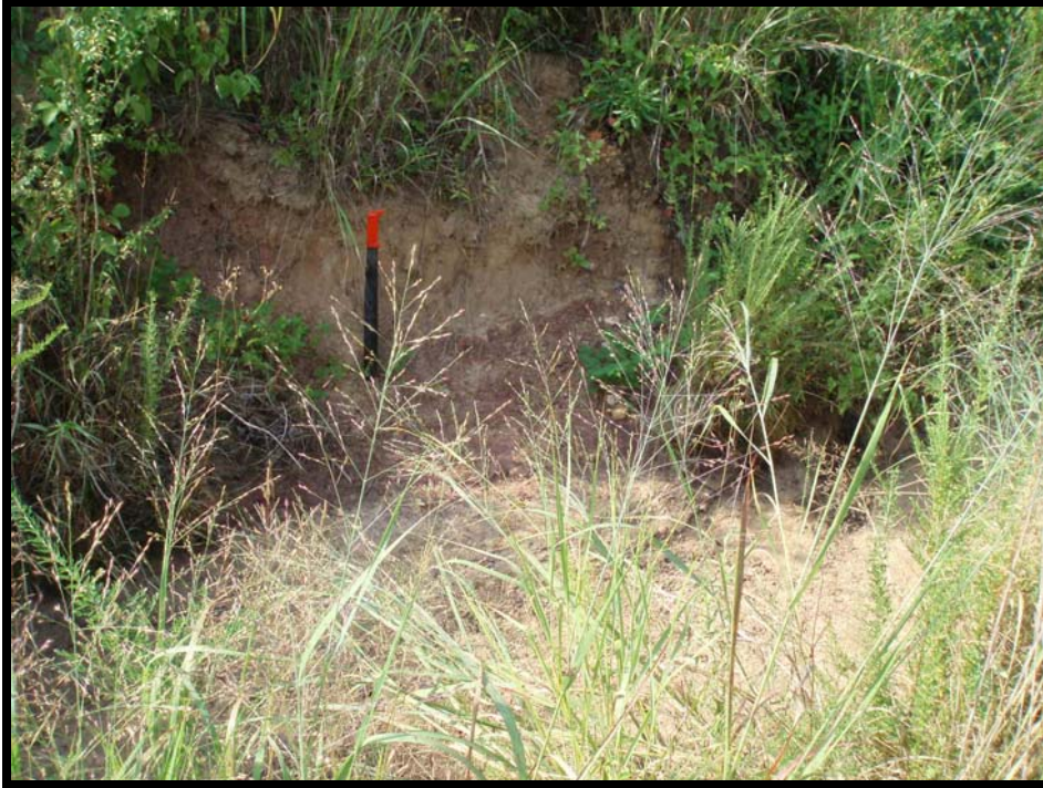
SPA3 - Left bank erosion and loss of vegetation @ station 16+30 (R1)
