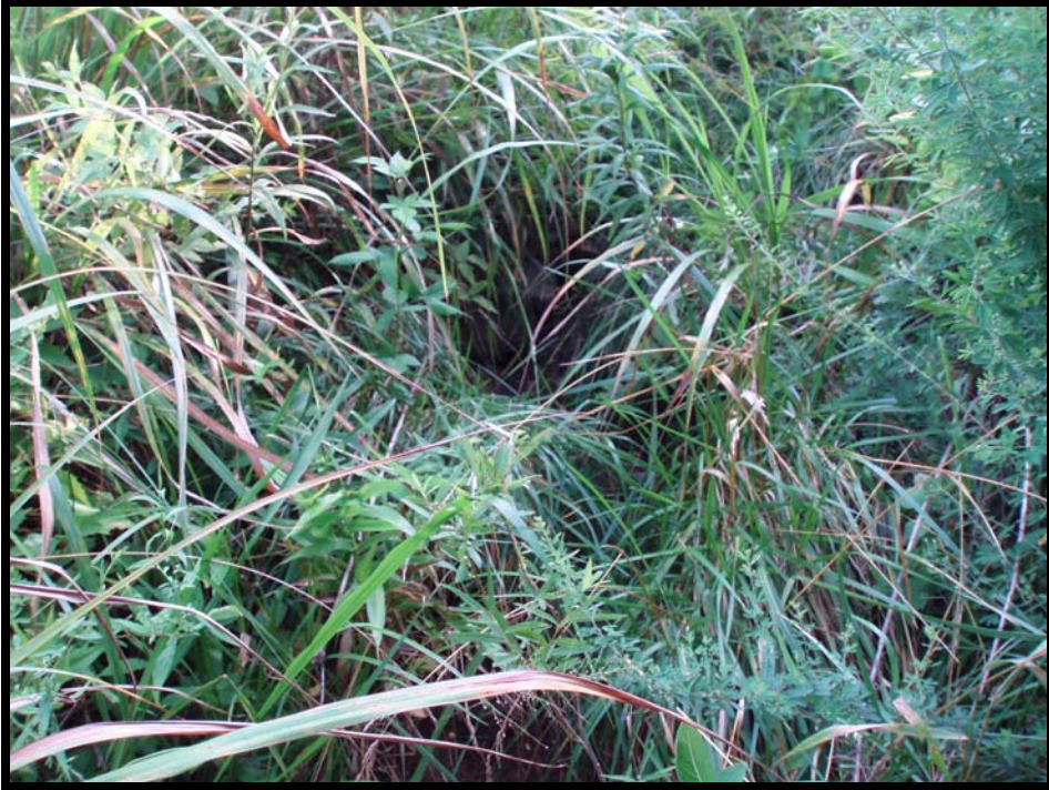
SPA1 - Small head cut in channel @ station 11+50 (R1)
