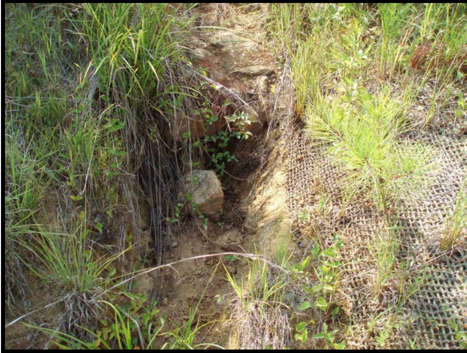
SPA10 - Erosion behind rock vane structure @ station 15+85 (S1)
