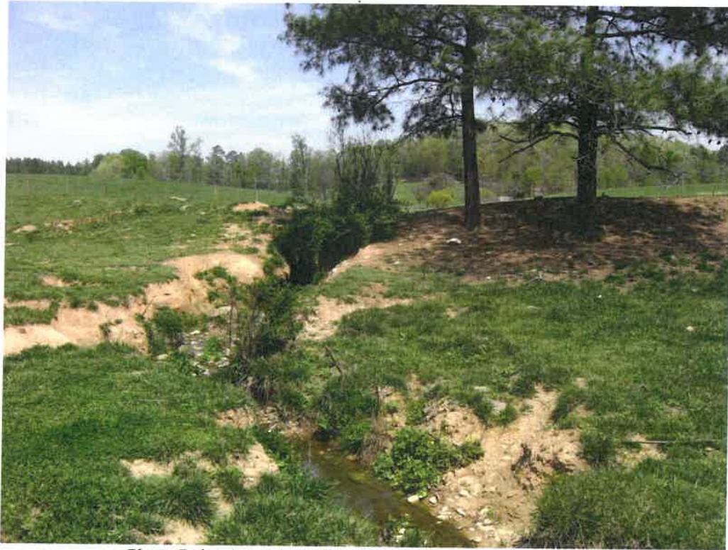
Photo Point 7: Looking Upstream (at breached farm pond)
