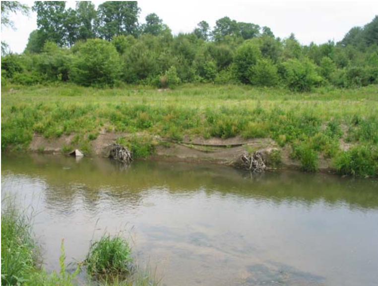
Photo 4 Bank instability at Station 1+00. Insufficient toe protection and too few root wads allowed steepening of the bank at this point.
