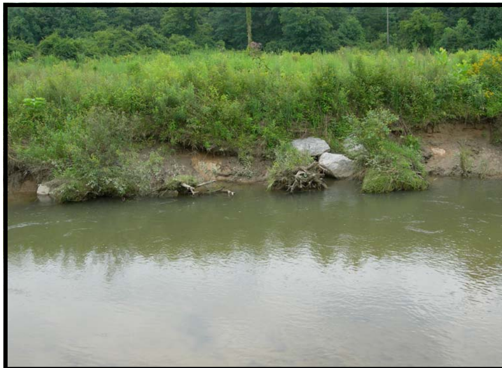
Photo 2—Representative Bank Scour/Stressed or Failing Structure
