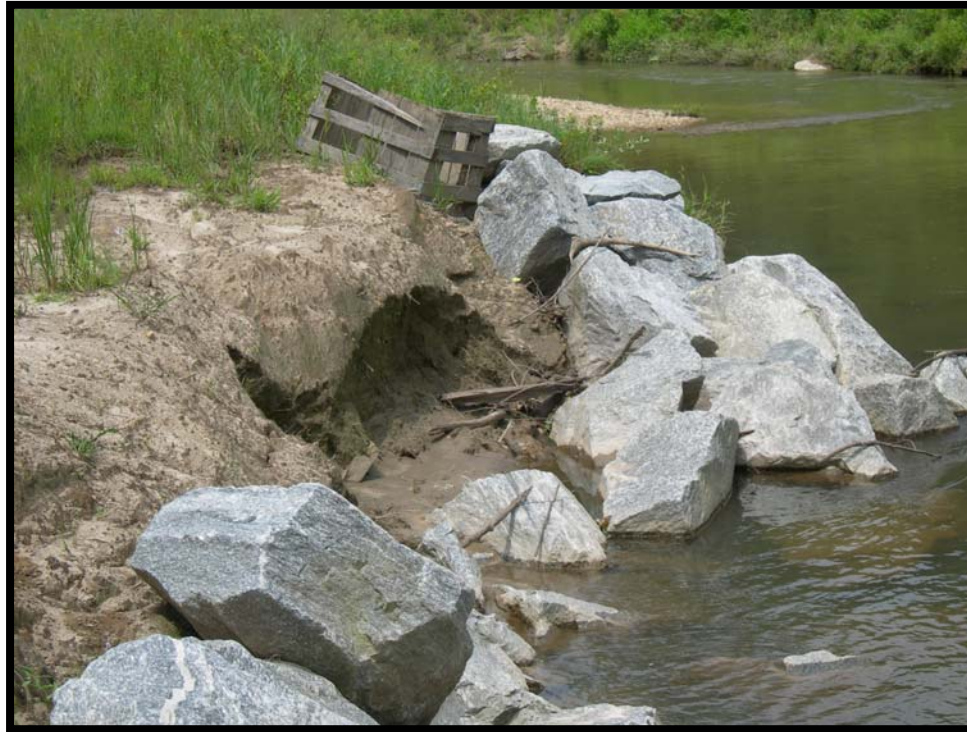
Photo 1—Representative Bank Scour
