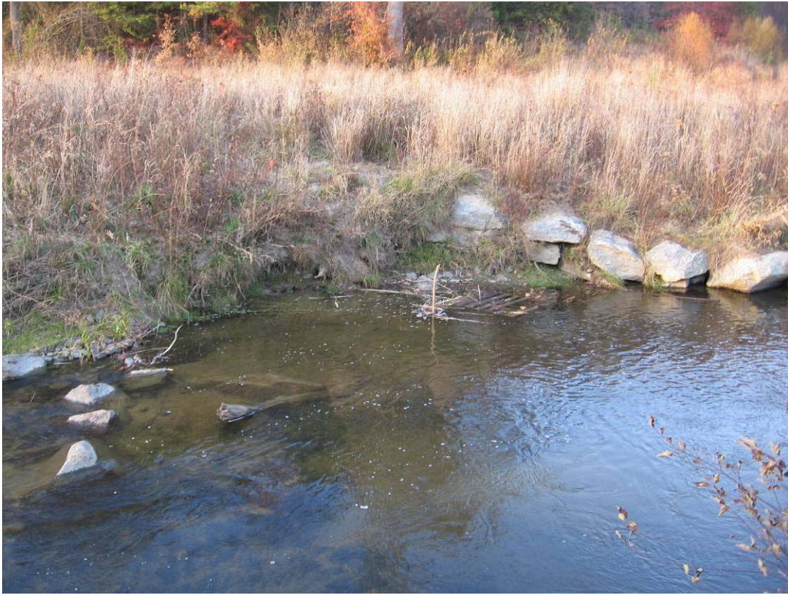
SP 1 – Looking upstream, bank scour on right bank downstream of structure arm
