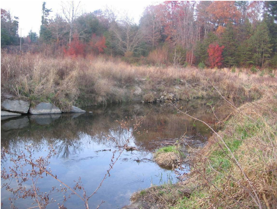
SP 6 – Looking upstream, scour of right bank and scour of root wads of right bank
