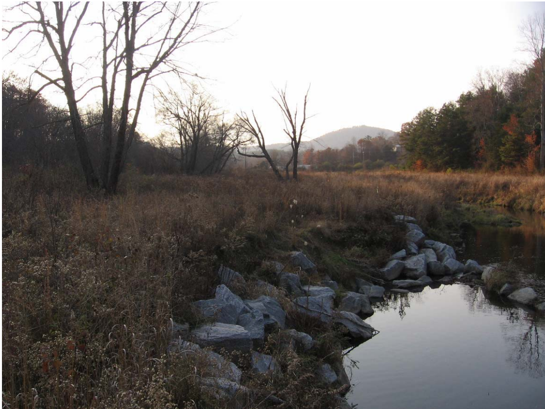
SP 4 – Looking downstream, collapse of rock used for bank protection
