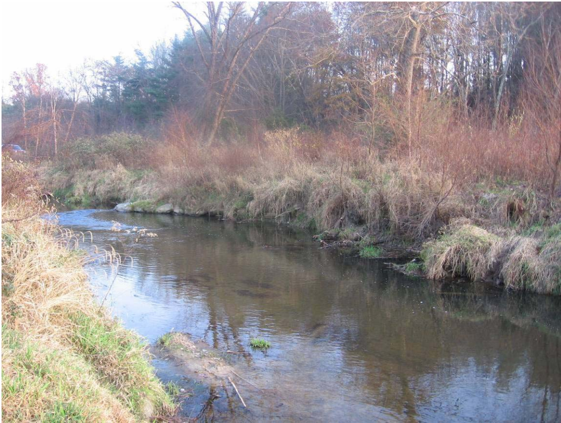
SP 2 – Looking upstream, bank scour on left bank downstream of structure arm
