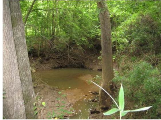
Photo 5 - Scour just downstream of sewer crossing
