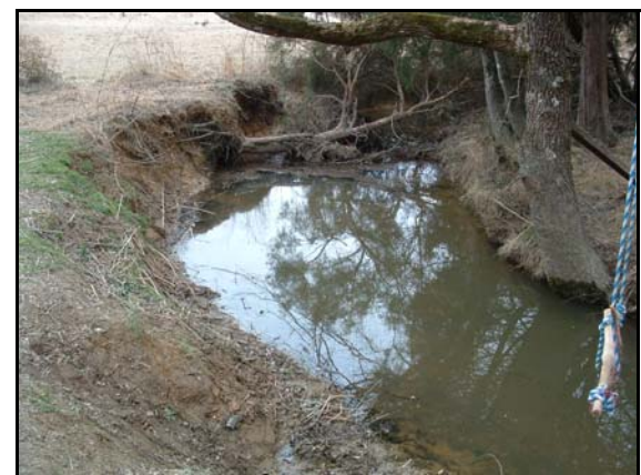
Eroding banks on the UT to Collins Creek when looking downstream.
