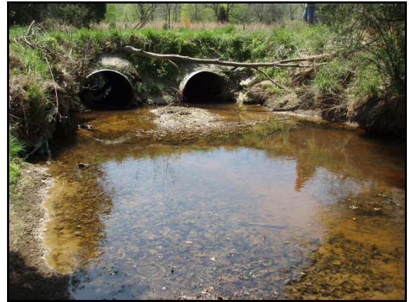
Looking downstream on UT to Collins Creek as it enters two culverts and crosses under a private road.
