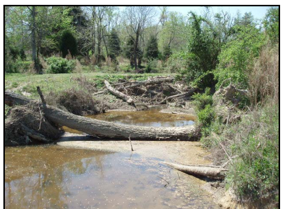
A look at the upstream side of a culvert on UT to Collins Creek that has become jammed with debris.
