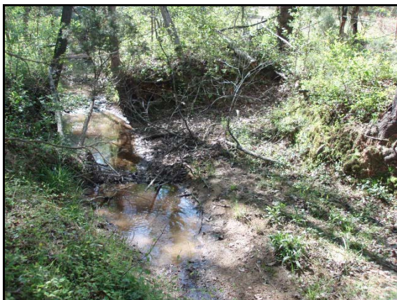
Looking downstream of the culvert where the channel of Tributary 1 has become too wide.
