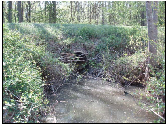
The beginning of Tributary 1 as it exits a culvert under Dodsons Crossroads.
