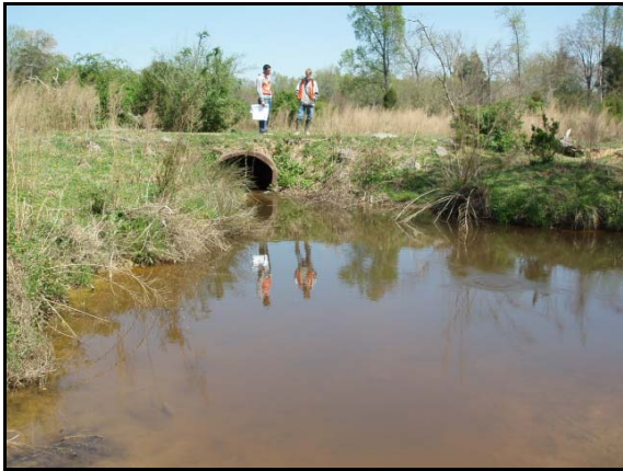
The downstream view of the jammed culvert along UT to Collins Creek. Water is currently working its way over the top of the crossing during bankfull events.
