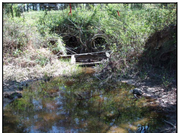
The beginning of Tributary 1B as it comes under Dodsons Crossroads through two culverts.
