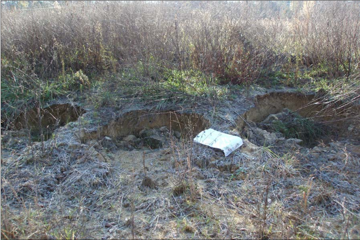
SP1 – Floodplain erosion taken near Station 107+00. 11/24/08 - MY 01
