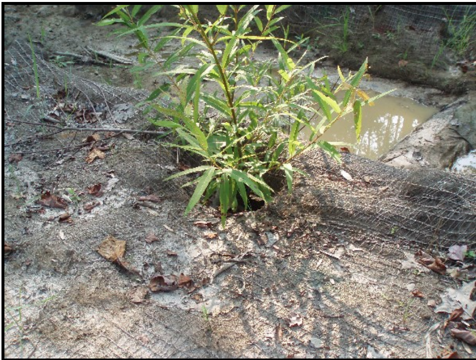
SPA 2. STA 12+30, erosion occurring behind log toe on log grade control.
