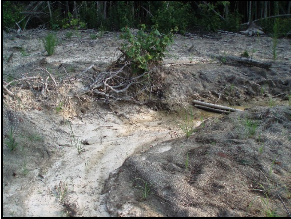
SPA 1. STA 20+60, erosion occurring on left bank on the downstream end of the log grade control.
