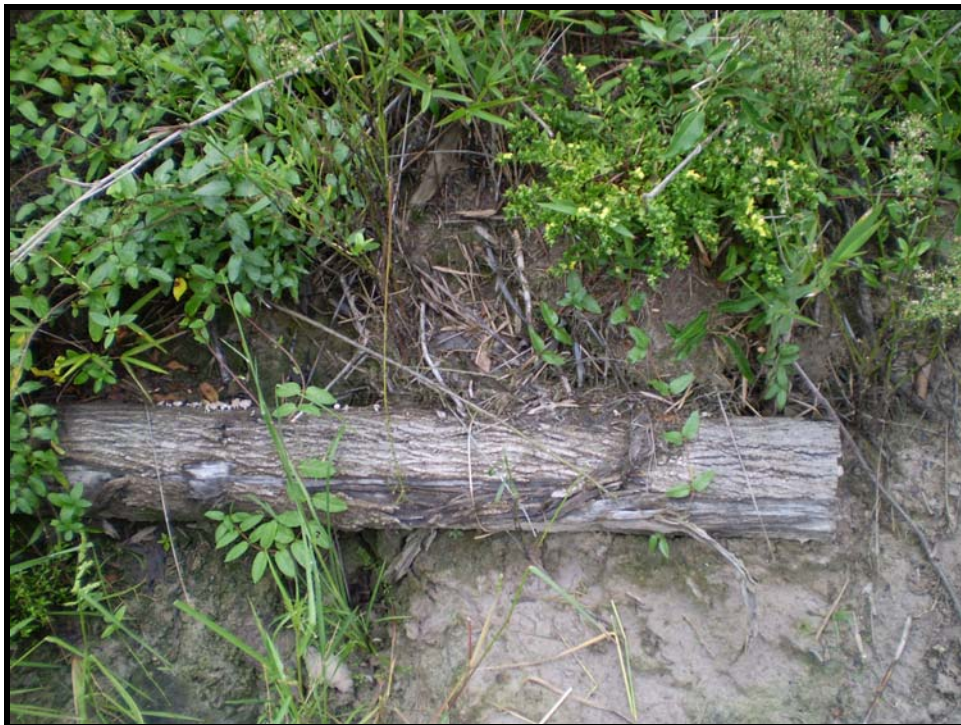
SPA 2. Erosion behind log toe on left bank at station 4+90.
