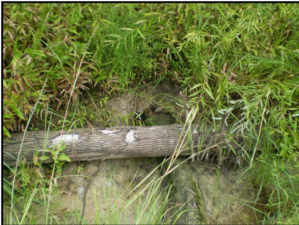
SPA 4. Right bank erosion behind log toe at station 22+20.
