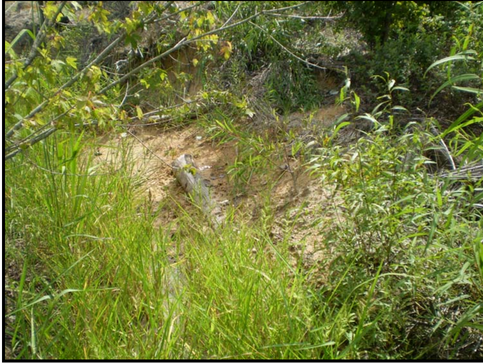
SPA 5. Right bank erosion behind log toe at station 35+75.
