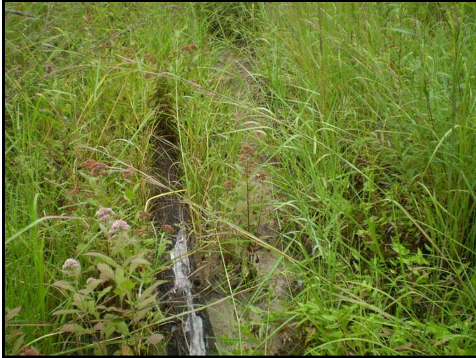
SPA 3. Scouring around log toe at station 19+05.
