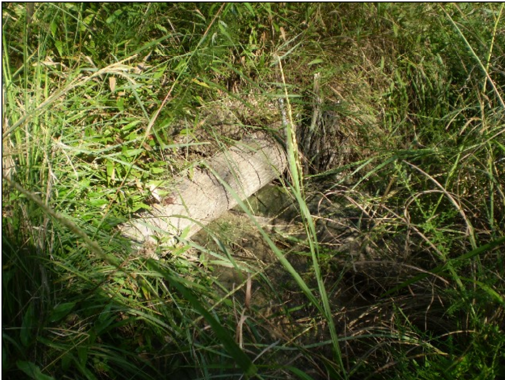
SPA 2. STA 22+20. Minor erosion on right bank at log grade control
