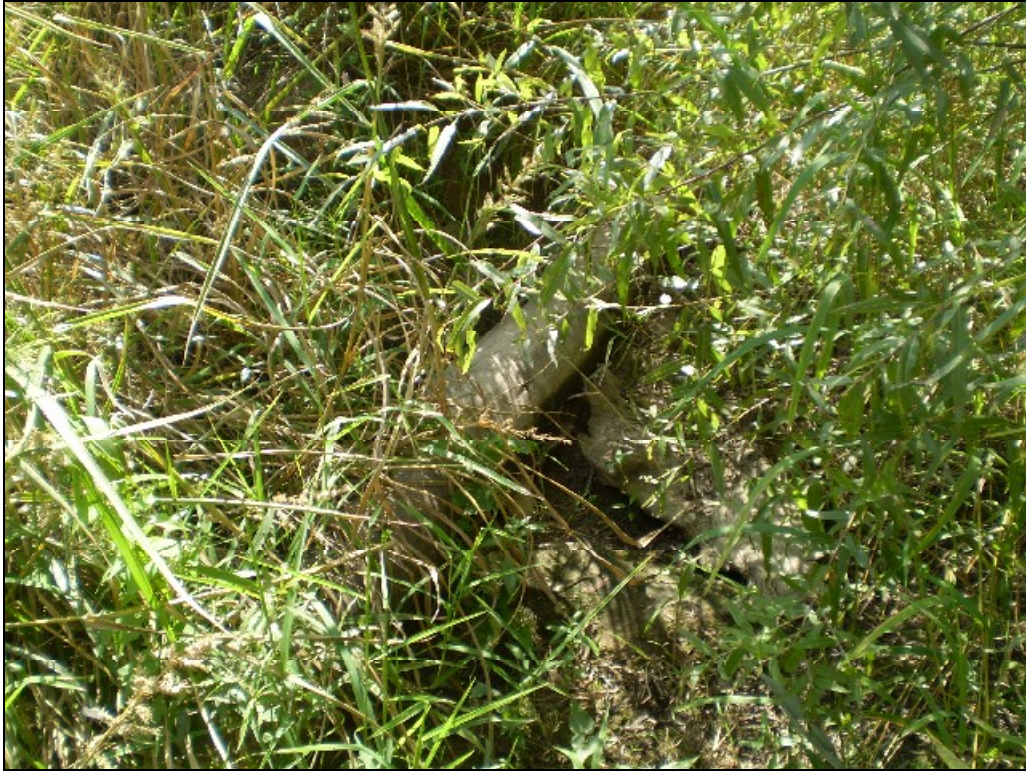
SPA 3. STA 34+80. Minor erosion behind log toe on left bank
