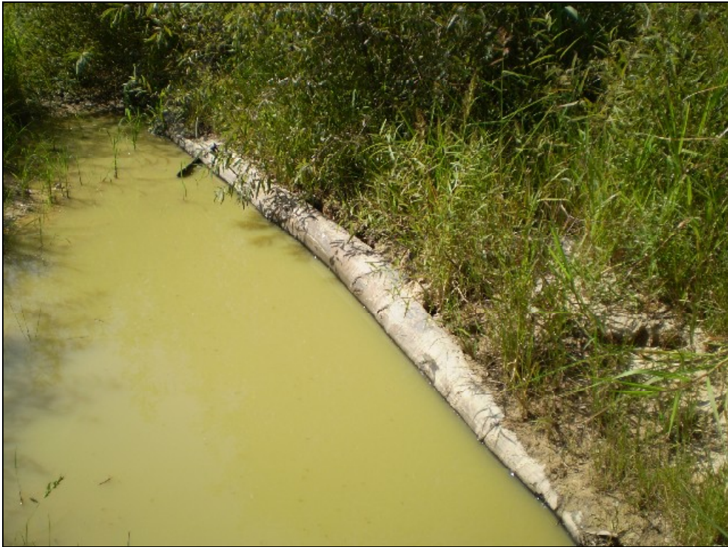
SPA 4. STA 45+30. Minor erosion behind log toe on right bank
