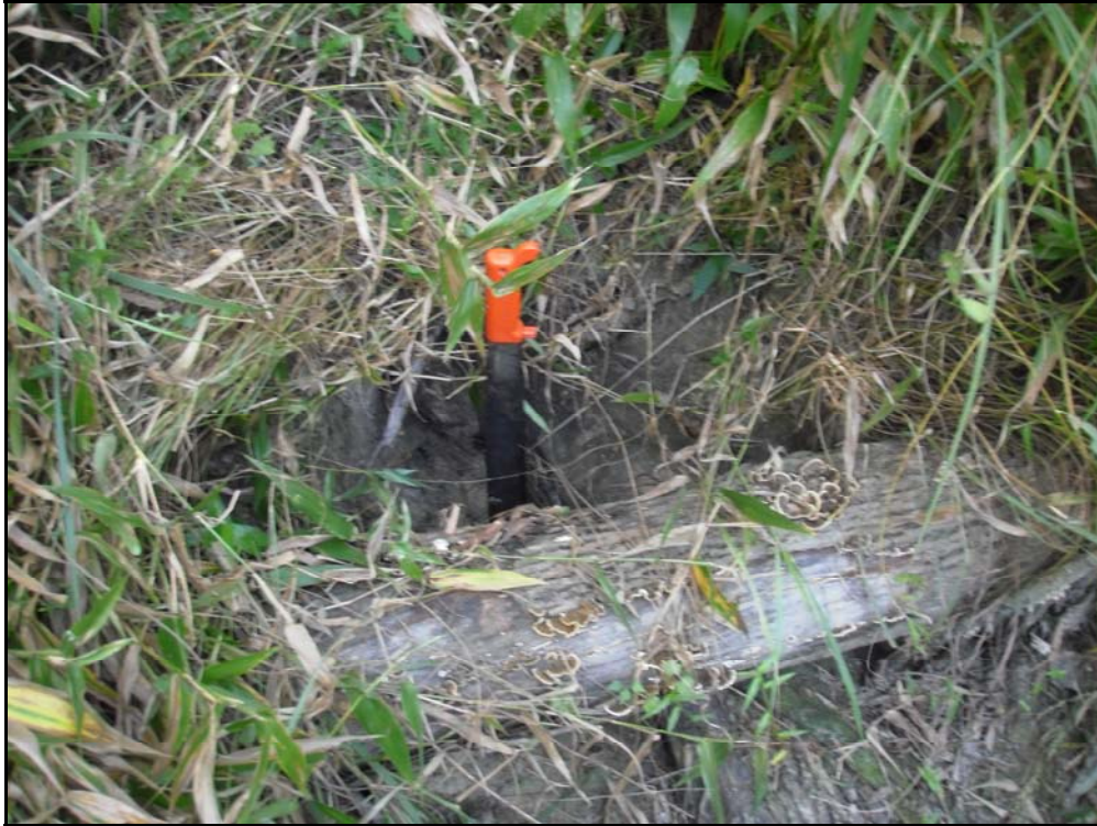
Photo #1 SOA Log Grade Control with erosion along left bank. Sta. 22+20
