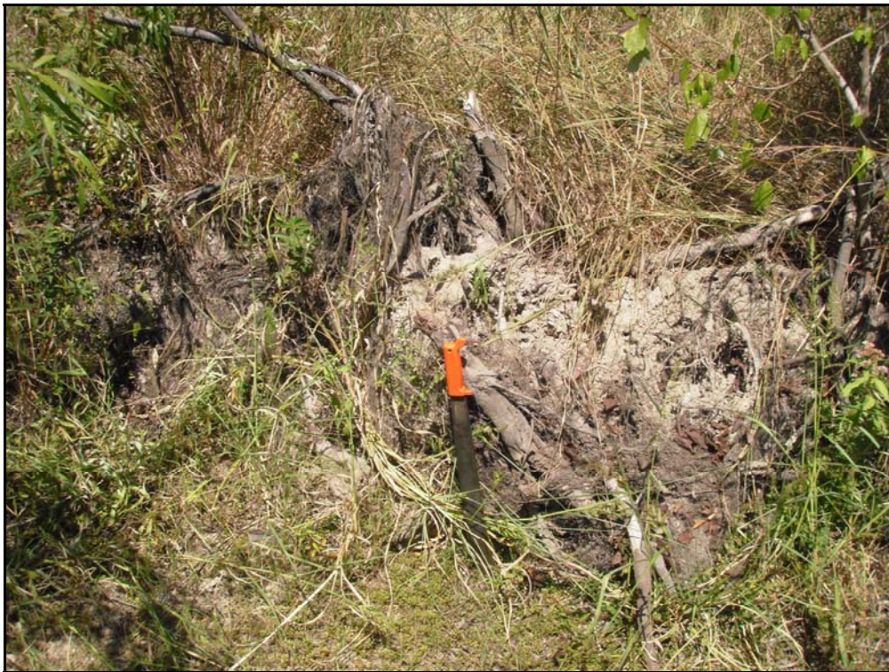
Photo #6 Rootwad, Sta. 27+60
