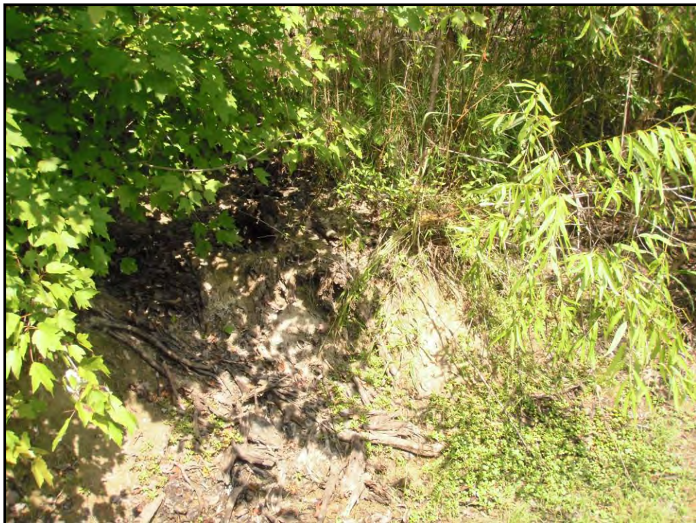
Photo #10 Rootwad, Sta. 36+30
