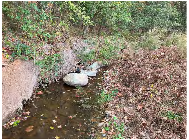
UT to Cedar Creek STA 127+74-128+44: Before – Dislodged Boulder Toe on Right Bank Causing Bank Erosion (11/10/2023)
