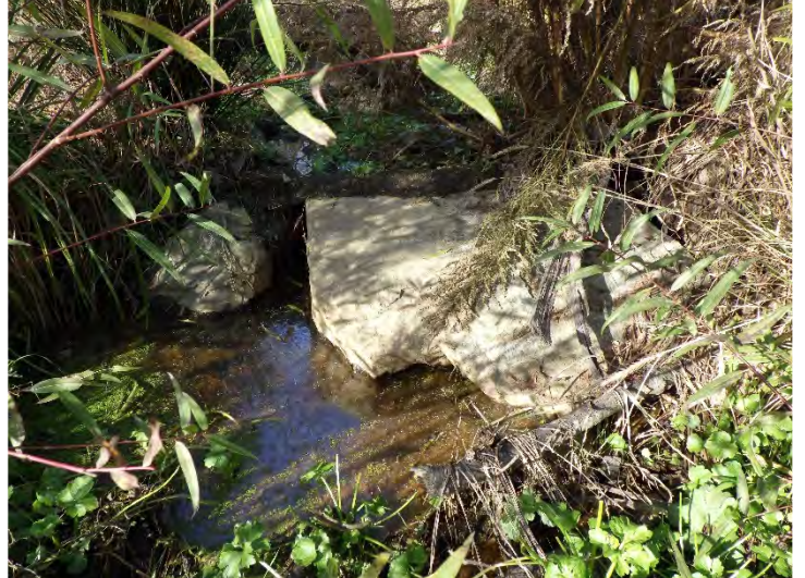
T8 STA 902+59: After –Piping Rock Sill Causing Localized Scouring (11/29/2023)
