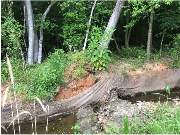
UT to Cedar Creek STA 127+74-128+44: Before – Partially Fallen Tree on Right Bank Causing Bank Erosion (4/7/2023)
