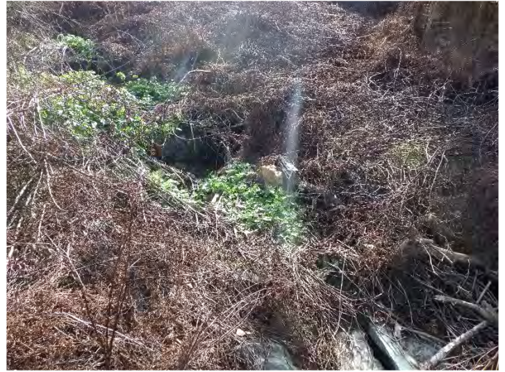
T2 STA 303+05-303+20: Before – Piping Log Sill Causing Dislodged Brush Toe and Scouring of the Left Bank (11/29/2023)
