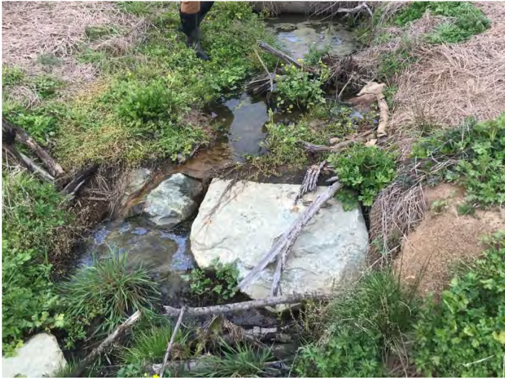
T8 STA 902+59: Before –Piping Rock Sill Causing Localized Scouring (4/7/2023)
