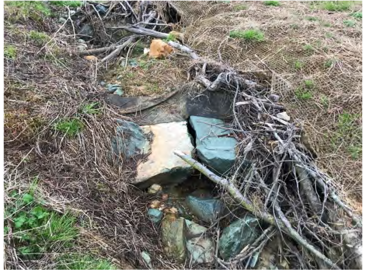
T2 STA 303+05-303+20: Before – Piping Rock Sill Causing Dislodged Brush Toe and Scouring of the Left Bank (4/7/2023)
