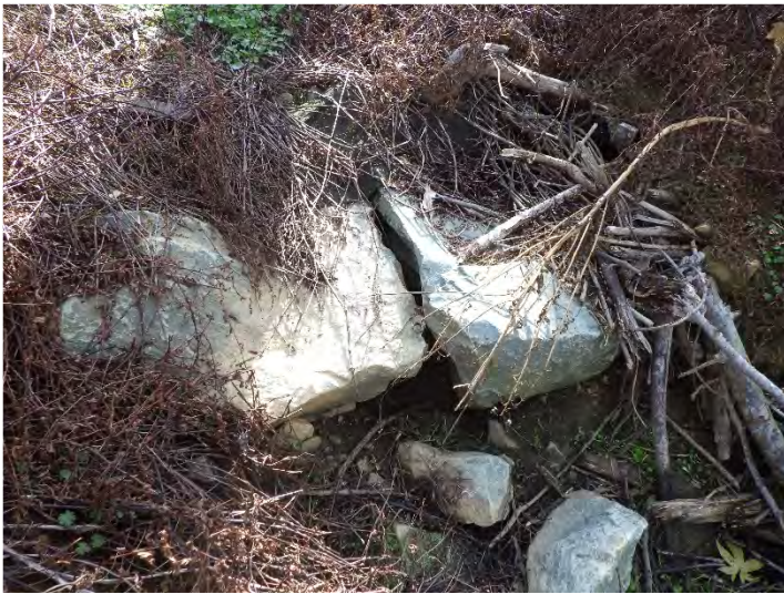
T2 STA 303+05-303+20: Before – Piping Rock Sill Causing Dislodged Brush Toe and Scouring of the Left Bank (11/29/2023)
