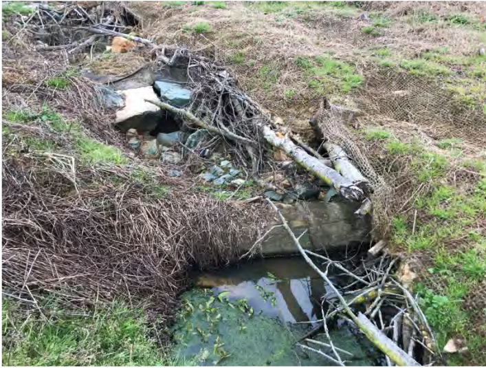
T2 STA 303+05-303+20: Before – Piping Log Sill Causing Dislodged Brush Toe and Scouring of the Left Bank (4/7/2023)
