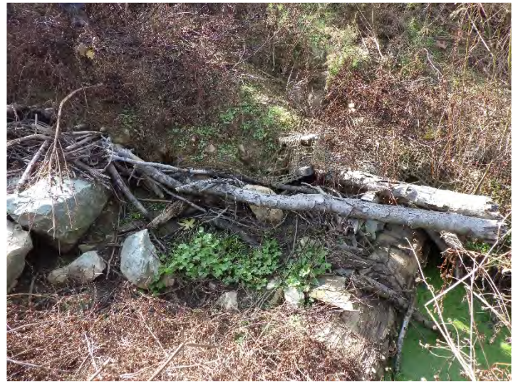
T2 STA 303+05-303+20: Before – Piping Log Sill Causing Dislodged Brush Toe and Scouring of the Left Bank (11/29/2023)
