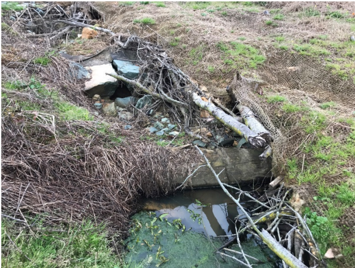
T2 STA 303+05-303+20: Before – Piping Log Sill Causing Dislodged Brush Toe and Scouring of the Left Bank (4/7/2023)
