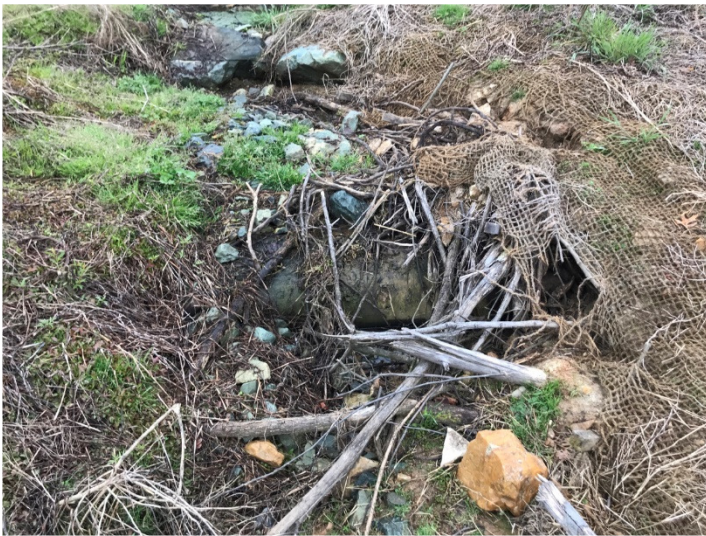
T2 STA 303+05-303+20: Before – Piping Log Sill Causing Dislodged Brush Toe and Scouring of the Left Bank (4/7/2023)
