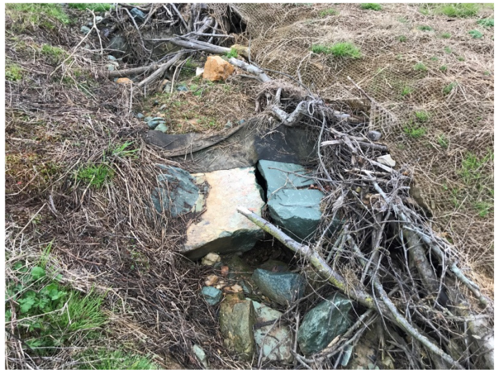
T2 STA 303+05-303+20: Before – Piping Rock Sill Causing Dislodged Brush Toe and Scouring of the Left Bank (4/7/2023)
