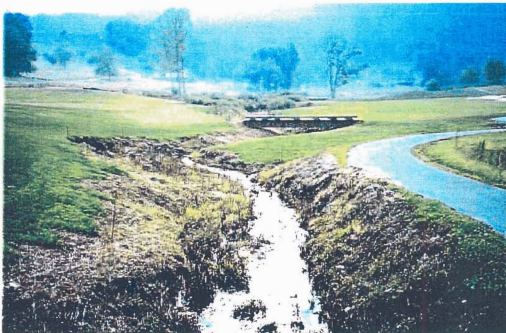
Photo 8: Looking upstream - eroded banks typical
