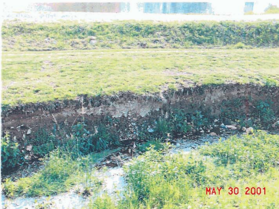
Photo 14: Severe erosion at greens
