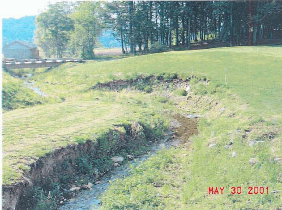
Photo 13: Eroded banks at 13 th green – looking d/s
