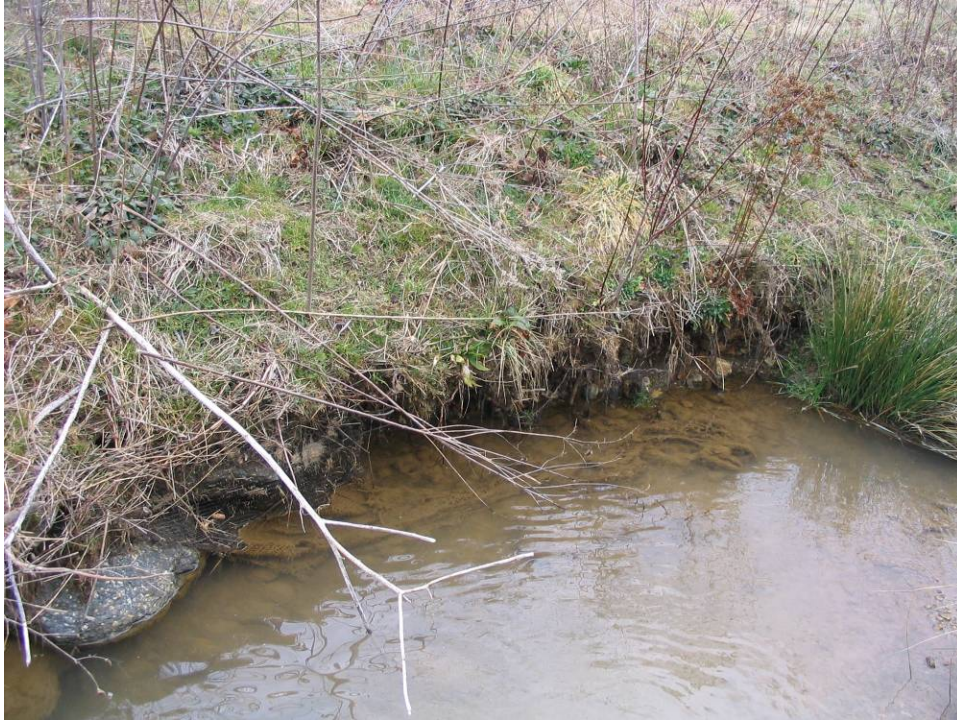
STA 32+00 Looking at Undercut Left Bank
