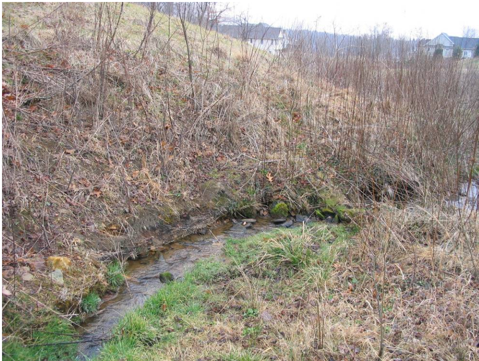
STA 9+10 Looking Downstream at Meander Bend and Bank Erosion
