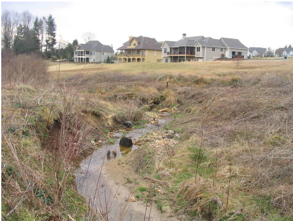
STA 29+30 Looking Downstream at Severe Bank Erosion on Left Bank and Head-Cut
