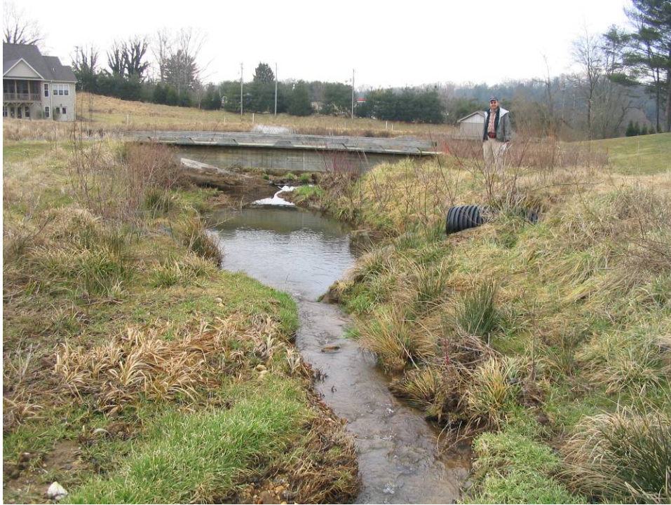
STA 32+90 Looking Downstream at Rock Cross Vane, Large Scour Pool, and 24" Storm-Water CPP
