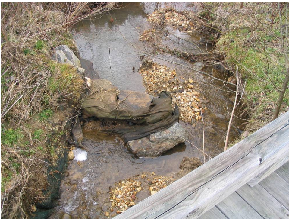
STA 35+00 Looking Down Stream at Failed Rock Cross Vane from Bridge
