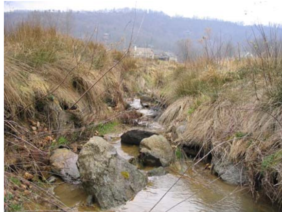
Issue Photo 2. Bank Erosion & Failed Rock Vane STA: 28+60
