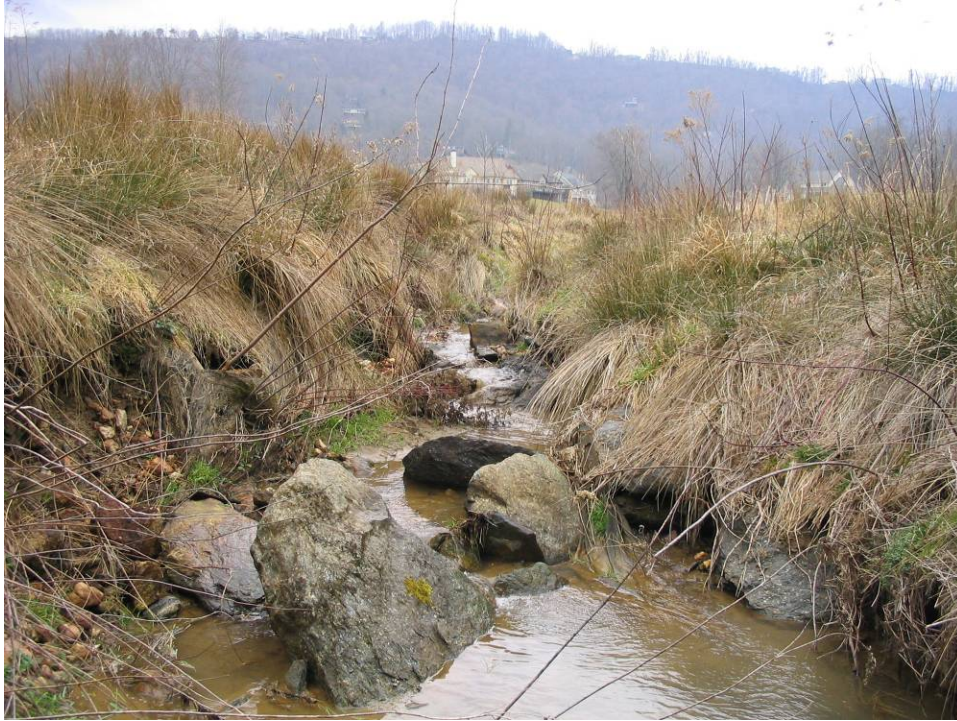
STA 28+50 Looking Upstream at Failed Rock Cross Vane
