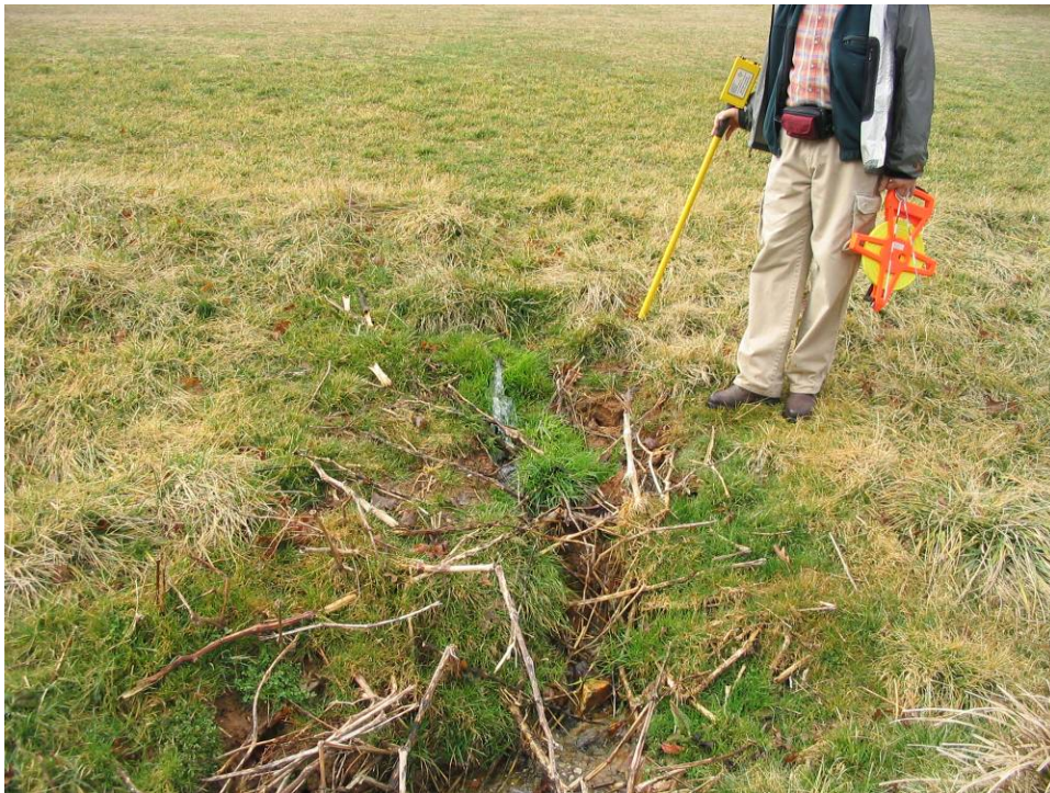
STA 11+40 Looking at Right Bank Upland Gully Erosion
