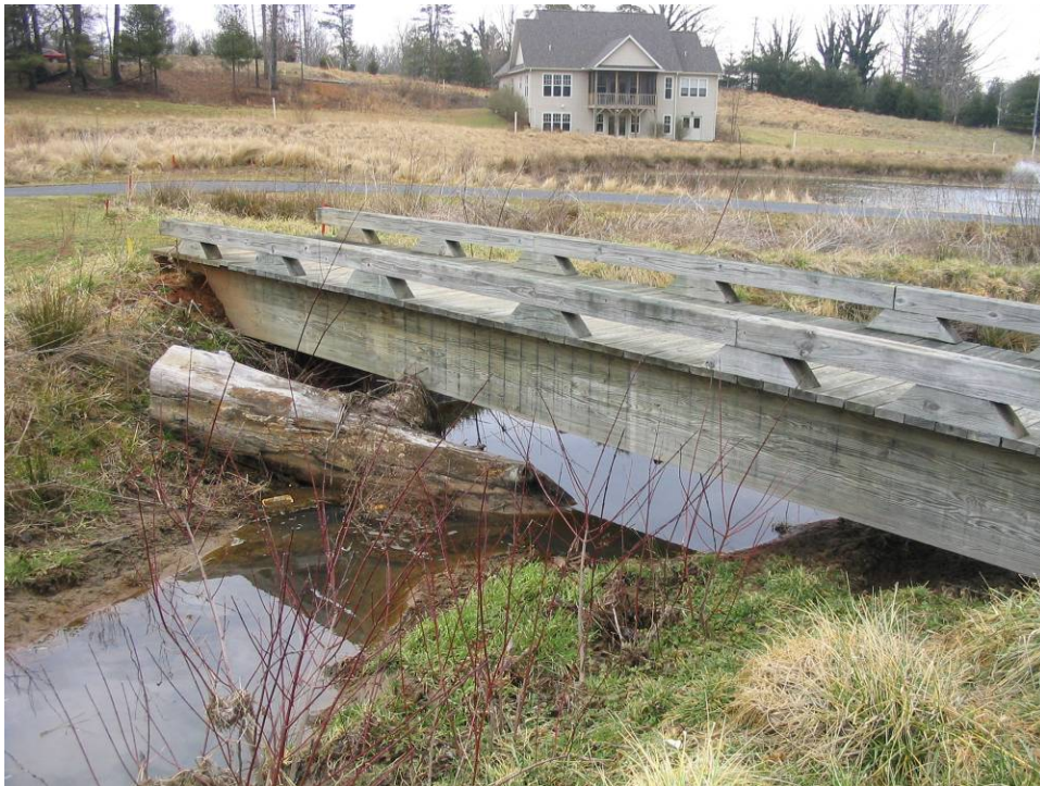
STA 33+30 Looking Downstream at Bridge and Log Debris Jam
