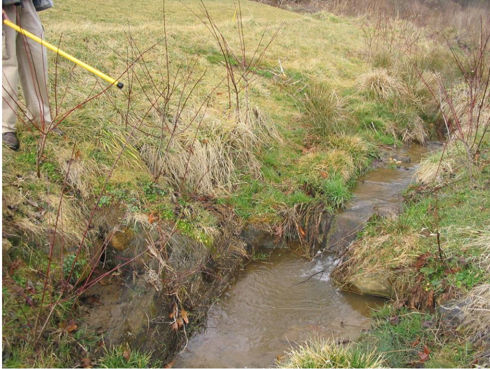
STA 11+50 Looking Upstream at Rock Cross Vane with Right Bank Erosion
