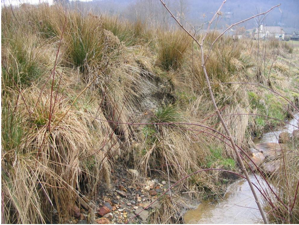
STA 28+20 Looking Upstream at Bank Erosion on Right Bank
