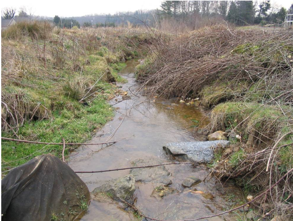
STA 28+75 Looking Downstream at Enlarged Channel and Failed Rock Cross Vane
