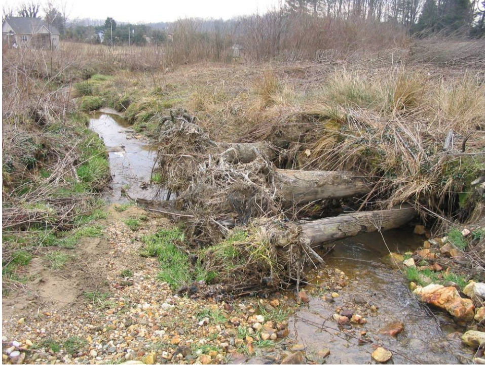
STA 29+90 Looking Downstream at Severe Head-Cut that has Exposed Root Wads
