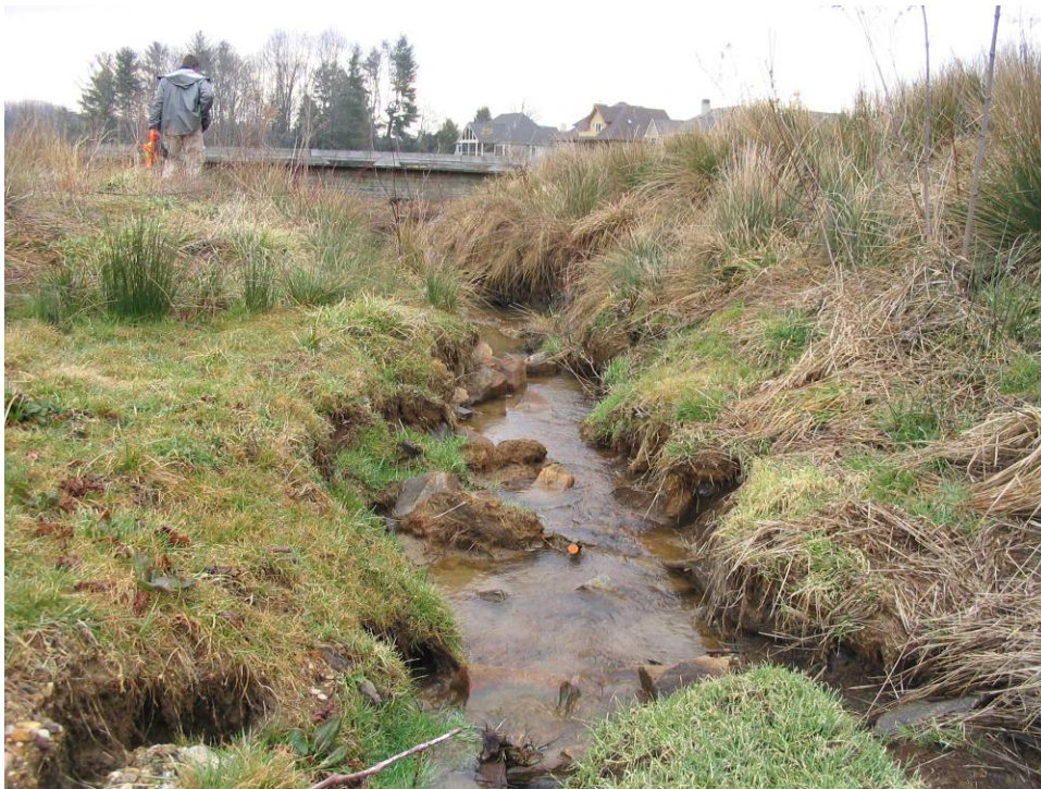
STA 27+75 Looking Downstream at Failing Rock Vane and Down-Cutting Channel
