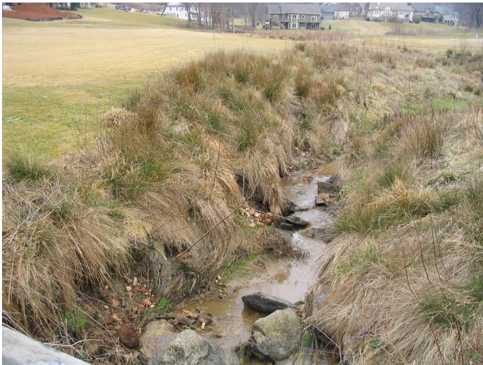
STA 28+60 Looking Upstream from Bridge at Down-Cutting and Failed Rock Cross Vanes
