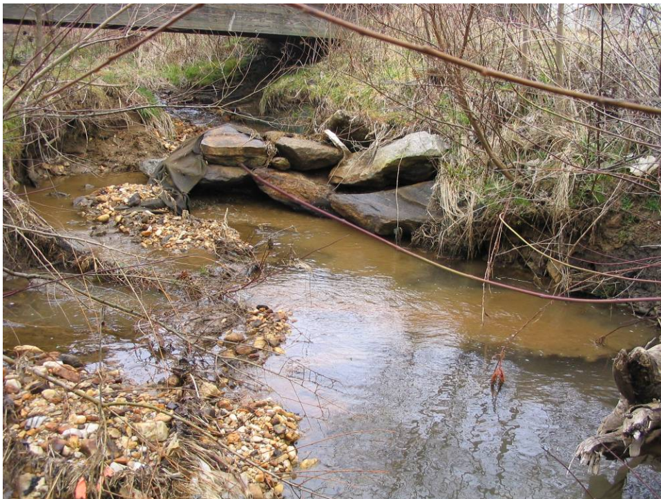
STA 35+20 Looking Upstream at Failed Rock Cross Vane
