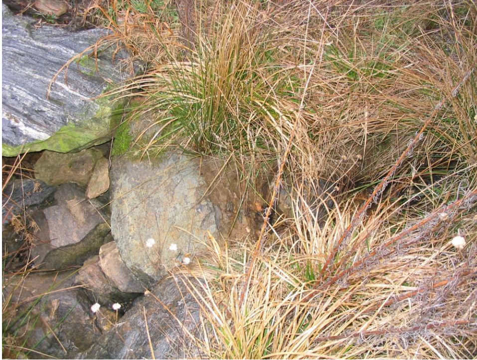
STA 3+70 Looking Upstream at Rock Cross Vane and Water Piping Through Vane
