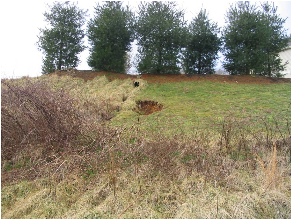
STA 14+40 Looking at Right Bank Hill Slope Erosion
