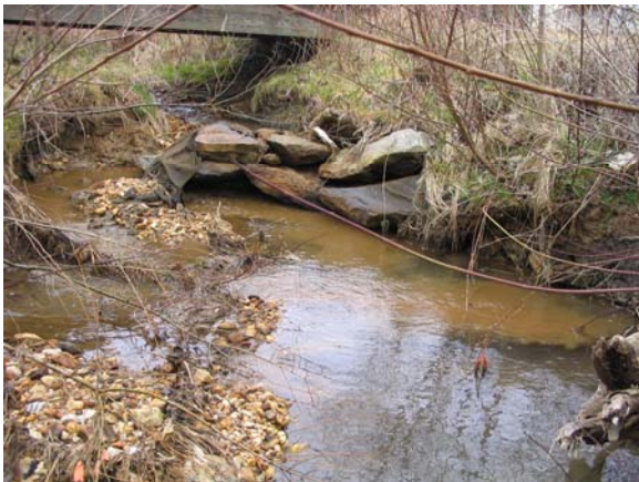
Issue Photo 1. Failed Structure STA: 35+10
