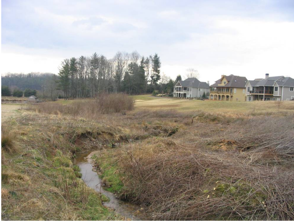
STA 29+10 Looking Downstream at Severe Bank Erosion on Left Bank
