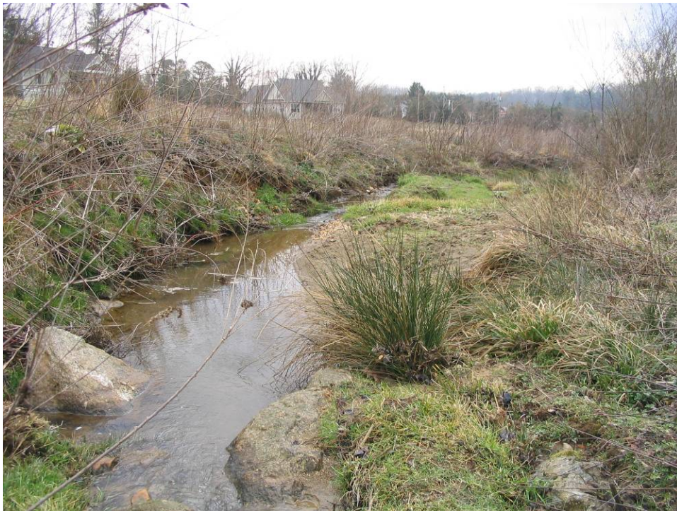
STA 31+40 Looking Downstream at Bank Erosion on Left Bank and Rock Cross Vane Holding Grade
