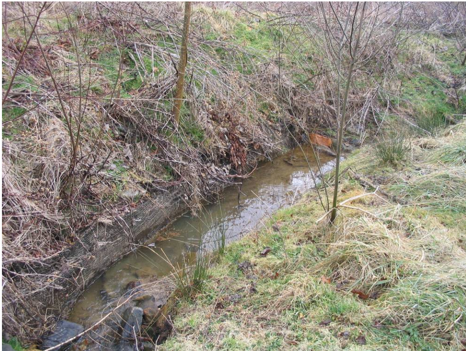
STA 15+50 Looking Downstream at Bank Erosion
