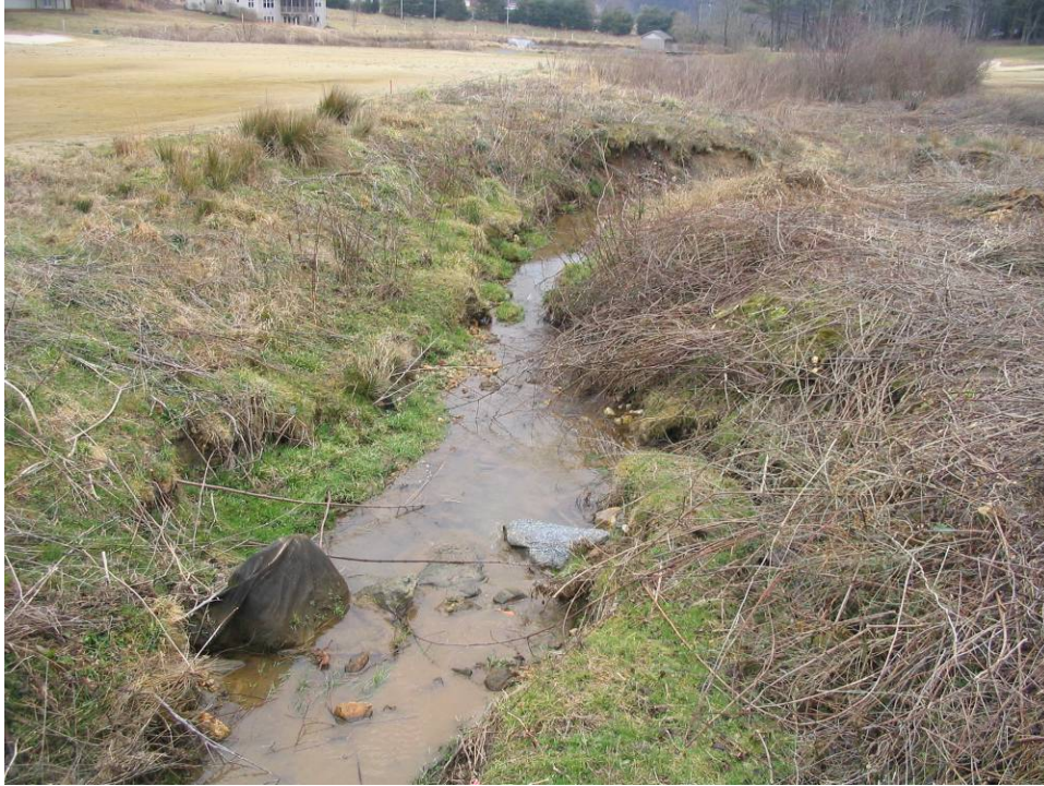
STA 28+70 Looking Downstream at Bank Erosion and Failed Rock Cross Vane
