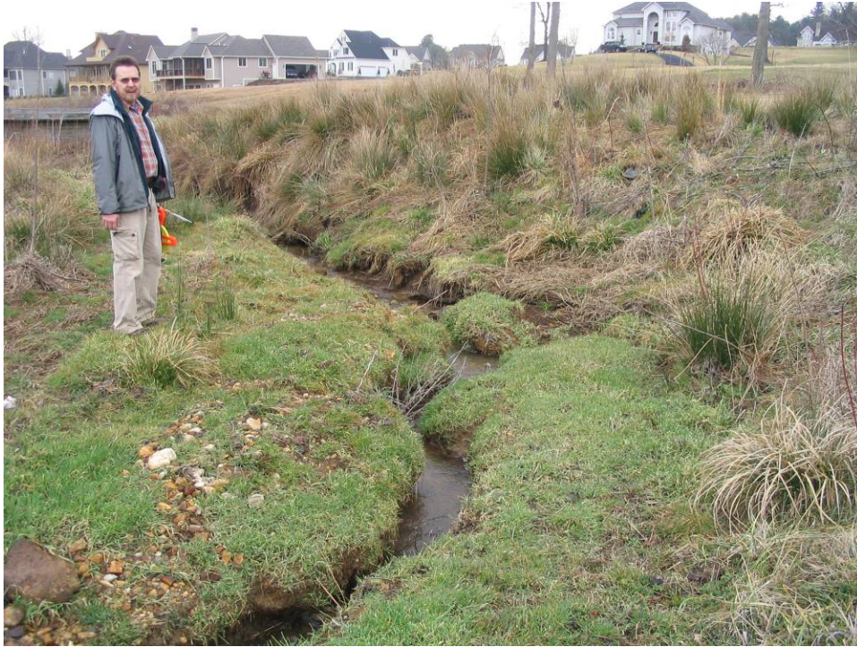
STA 27+60 Looking Downstream at Bankfull Bench Down-Cut
