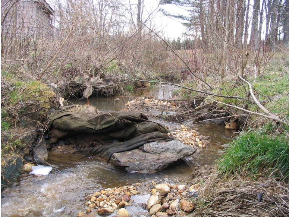
STA 35+00 Looking Down Stream at Failed Rock Cross Vane
