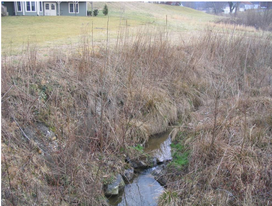
STA 22+80 Looking Upstream at Rock Vane with Confined Right Bank Erosion
