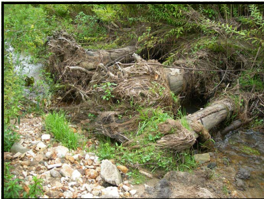
Figure 2— Typical Bank Scour / Failing Structure
