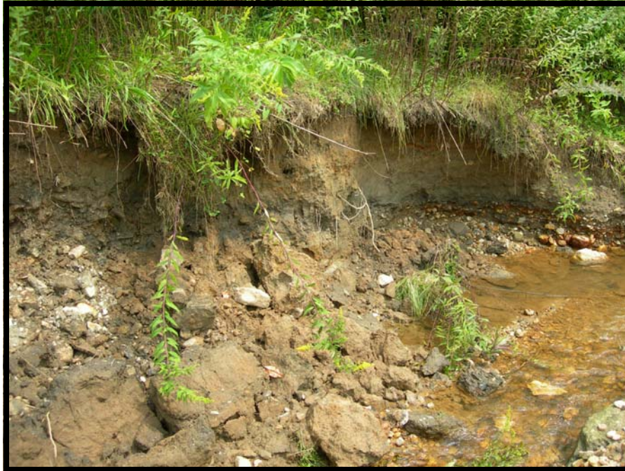
Figure 1— Typical Bank Scour
