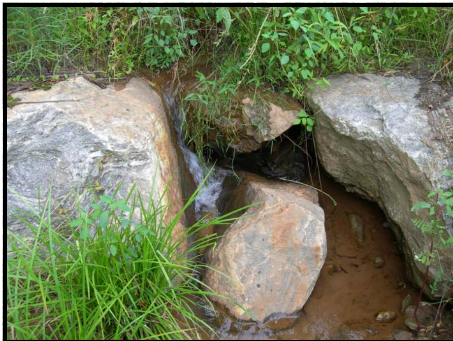
Figure 4—Typical Failing Structure
