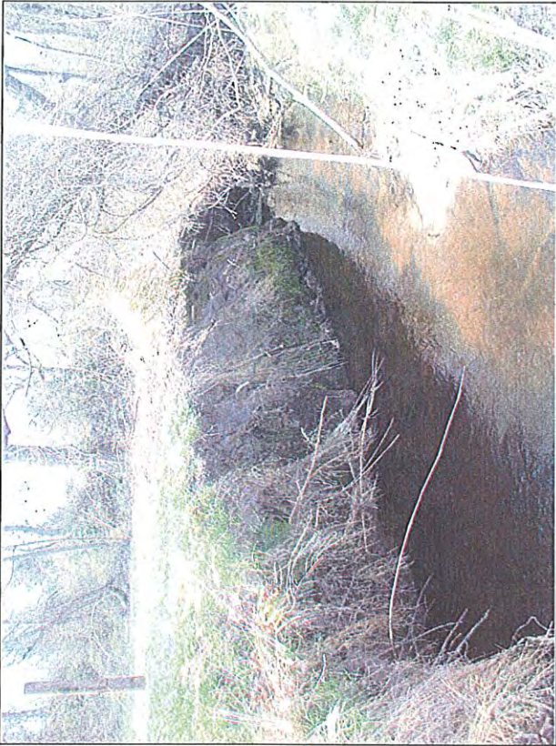
Bank Erosion in Cox Branch.
