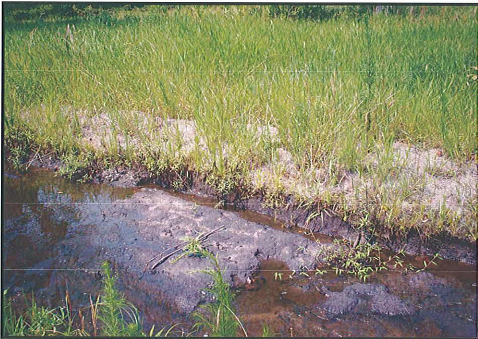
SPA 4. Left bank erosion at STA 52+70.
