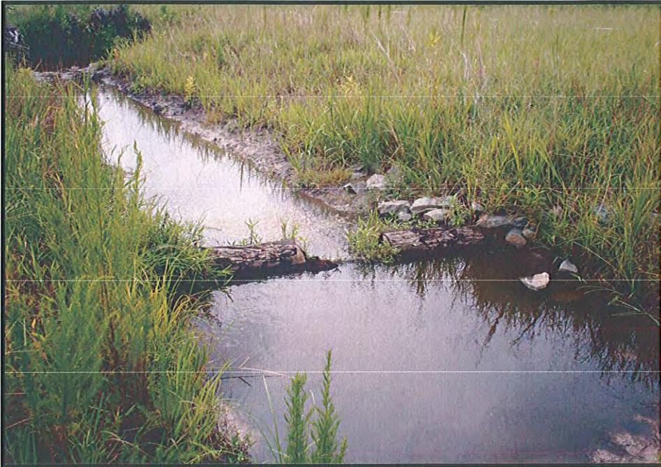
SPA 1. Undercutting at log weir STA 20+40 (repaired September 2006).
