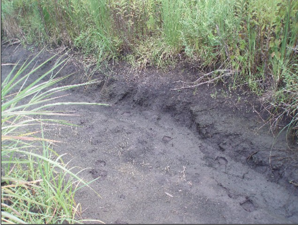
SPA #17. STA 74+50. Erosion on right bank downstream of log vane.
