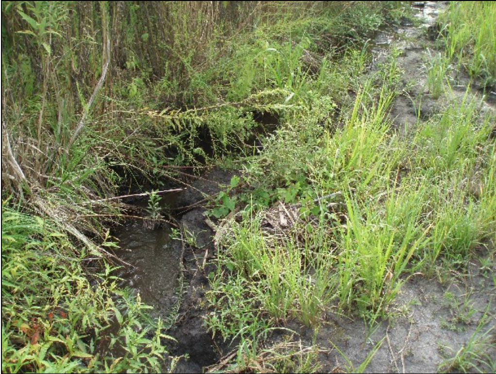
SPA #15. STA 66+40. Head cut and bed erosion.
