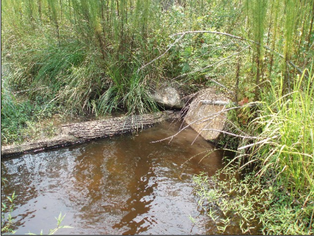
SPA #7. STA 46+80. Log weir undercut on left bank.
