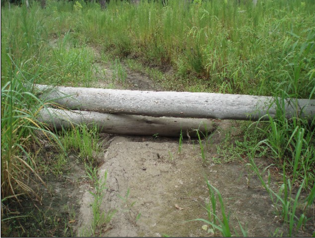
SPA #21. STA 82+80. Head cut and bed erosion.
