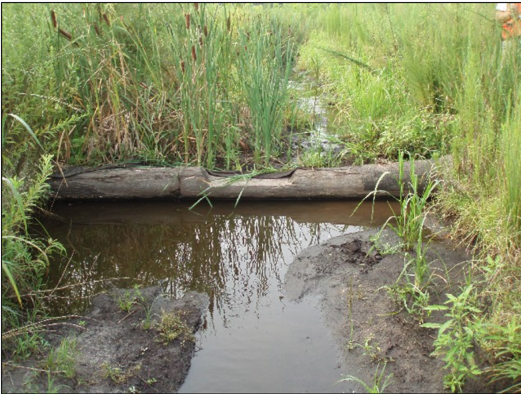
SPA #14. STA 65+30. Log weir end cut on left bank.
