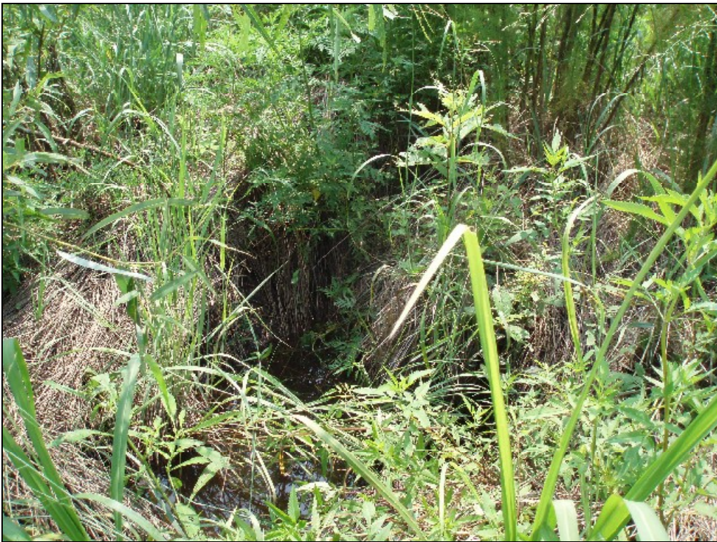
SPA #6. STA 37+00. Erosion on right bank.
