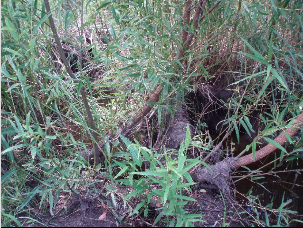
SPA #5. STA 33+70. Log weir end cut on left bank.
