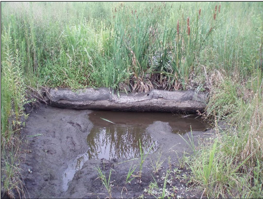
SPA #16. STA 71+40. Log weir undercut.
