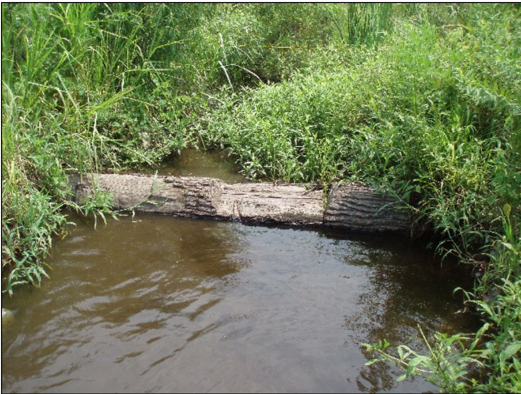
SPA #4. 31+40. Log weir undercut on right bank.
