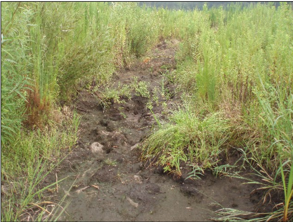
SPA #18. STA 74+80. Bed erosion.
