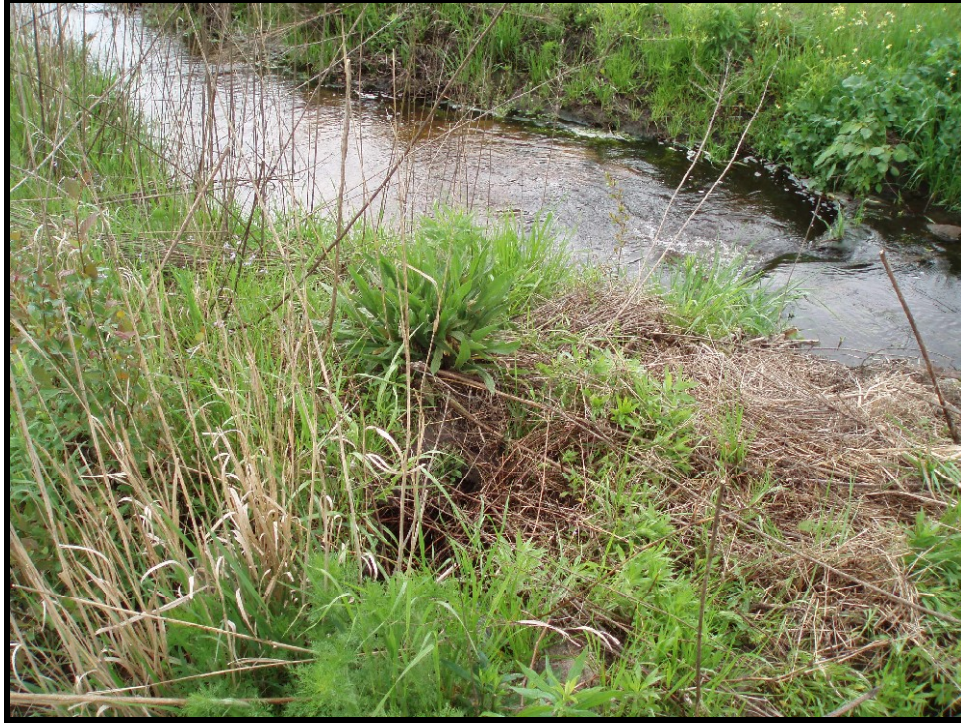
SPA3. Sta. 20+40 End cut on right bank due to improper installation of log weir; bed stable.
