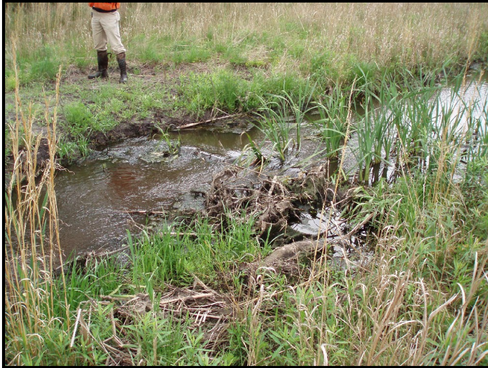
SPA9. Sta. 57+10 Erosion on left bank at log weir; end cut on right bank has been repaired.
