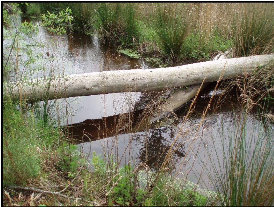
SPA14. Sta. 84+00 Log in channel directing flow to sides of channel, causing minor erosion.
