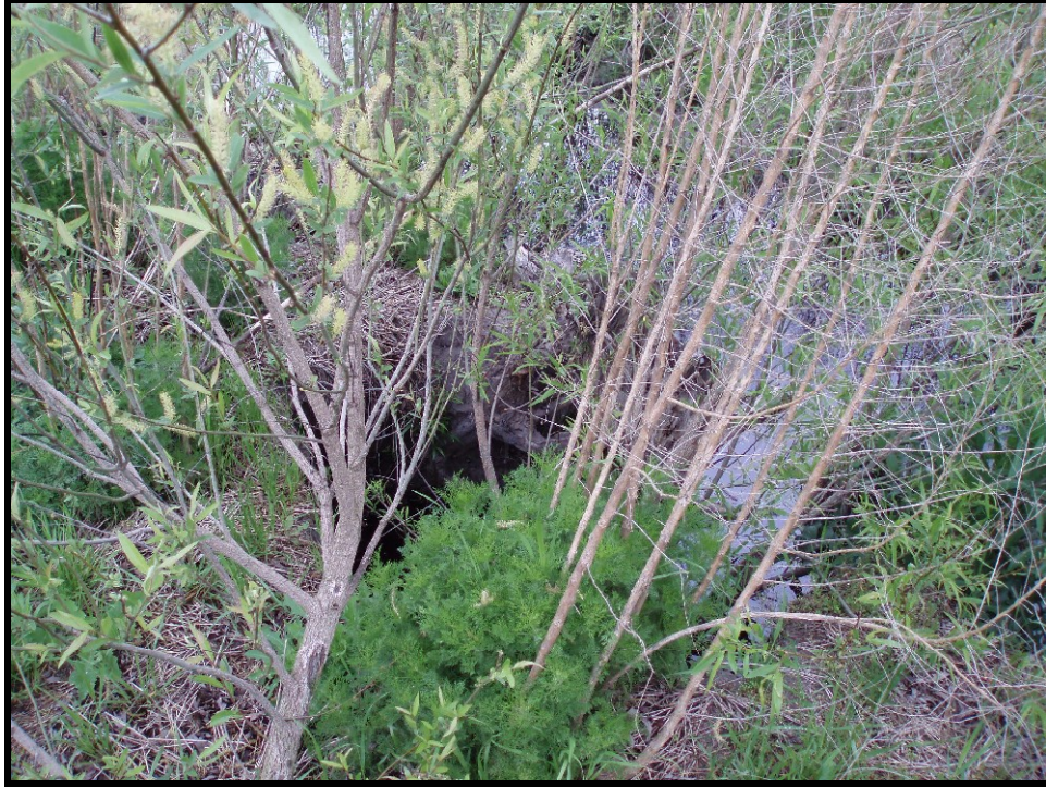
SPA5. Sta. 23+50 Erosion behind root wad on downstream end; other root wads are stable.
