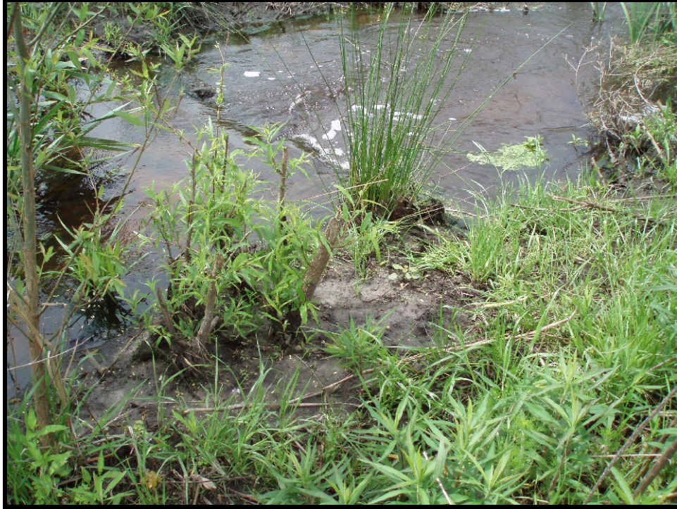
SPA7. Sta. 31+40 Undercut on right bank at log weir; banks appear stable.
