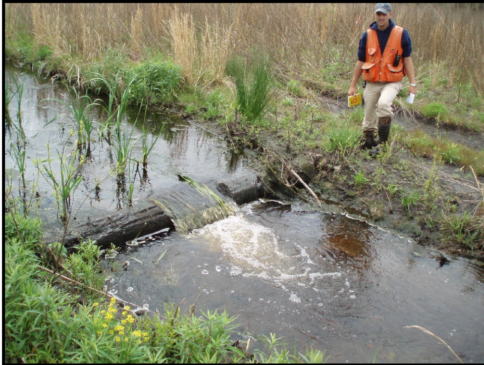
SPA10. Sta. 65+30 Undercut on left bank at log weir; has been repaired, but is still eroding.
