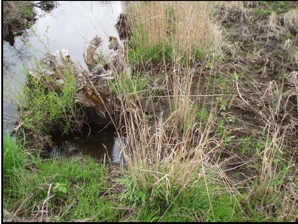
SPA1. Sta. 18+00 Erosion on right bank behind root wads.
