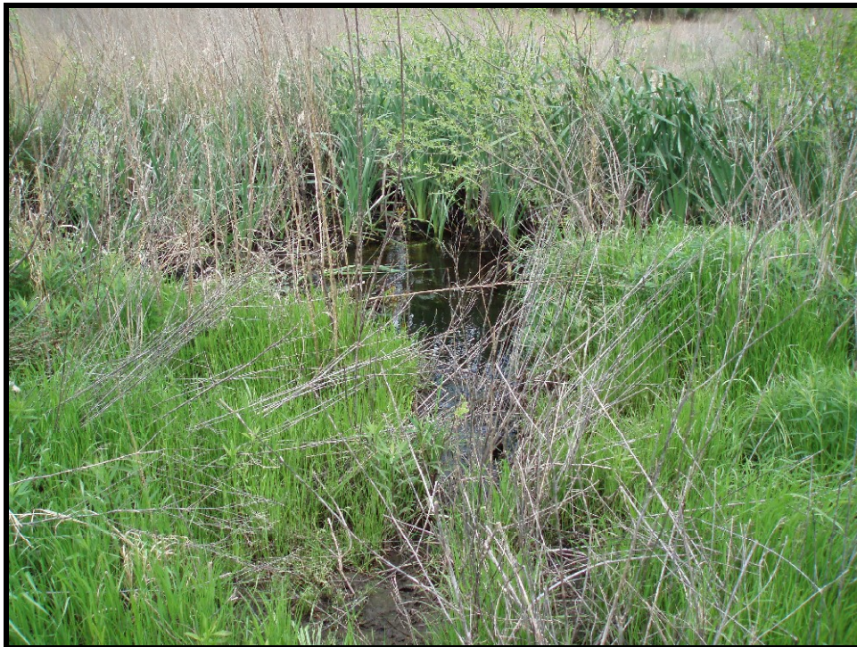
SPA8. Sta. 37+00 Minor right bank erosion at channel plug.
