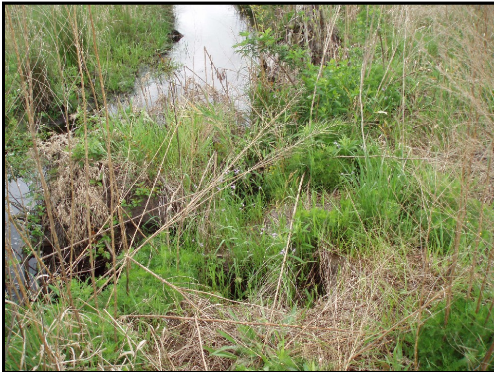
SPA2. Sta. 20+00 Erosion on right bank behind root wads.
