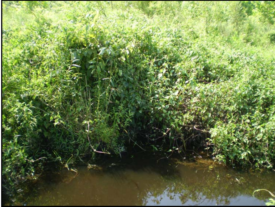
SPA 1 - Erosion behind root wads, Sta. 18+00.
