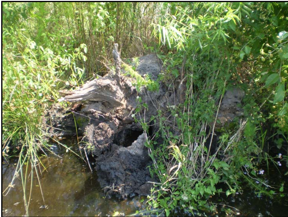
SPA 2 - Erosion behind root wads, Sta. 20+00.
