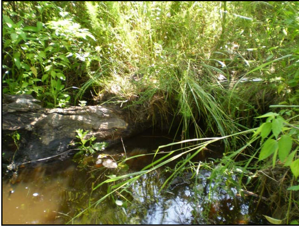
SOA 1 - Erosion on right bank behind root wads, Sta. 24+25.
