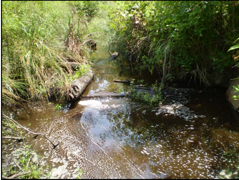
SOA 5 – Erosion on left and right banks at log weir, Sta. 46+85.
