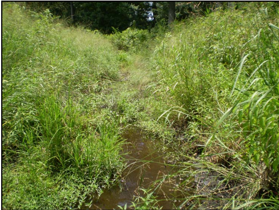
SOA 4 – Vegetation in channel, Sta. 45+50.
