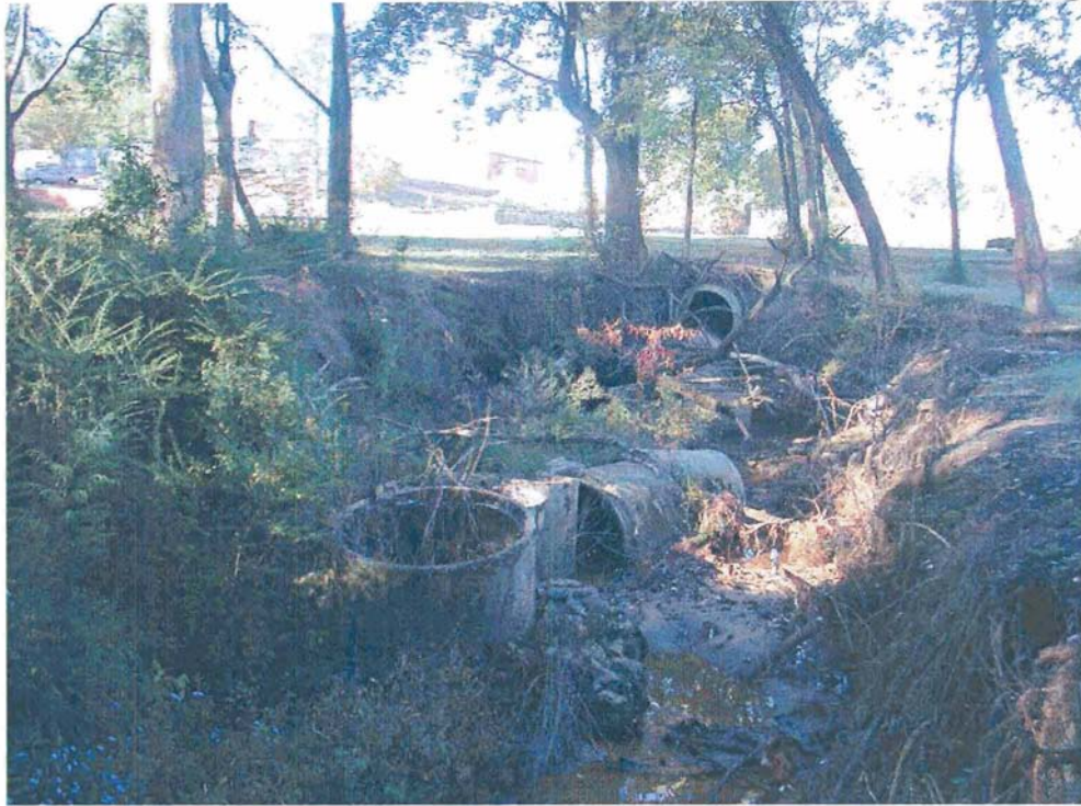
Picture 13. Large drainage ditch at south end of property. 48" pipe has failed .
