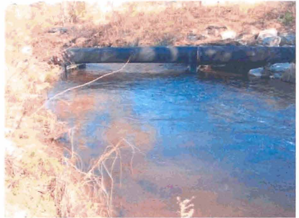
SPA 2. Station 15+80 Bowling effect caused by pool formation below utility pipe.
