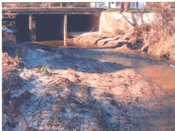
SPA 6. Station 10+50 on Little Cross Creek (LCC). Deposition causing point bar formation.
