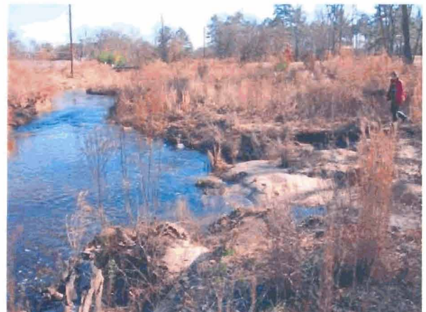
SPA 5. Station 21+50 Current state of outside meander; bank failure occurring.
